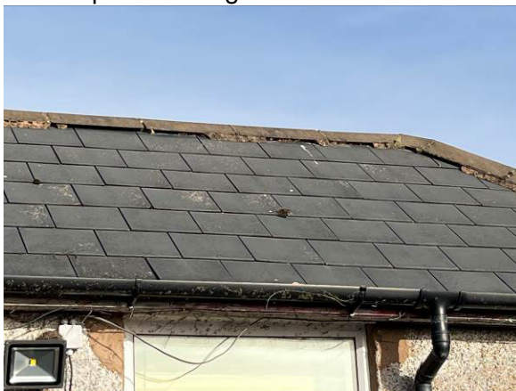
Gaps under ridge tiles on south side
