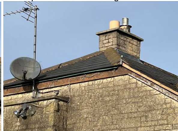
Gaps around chimney stack
