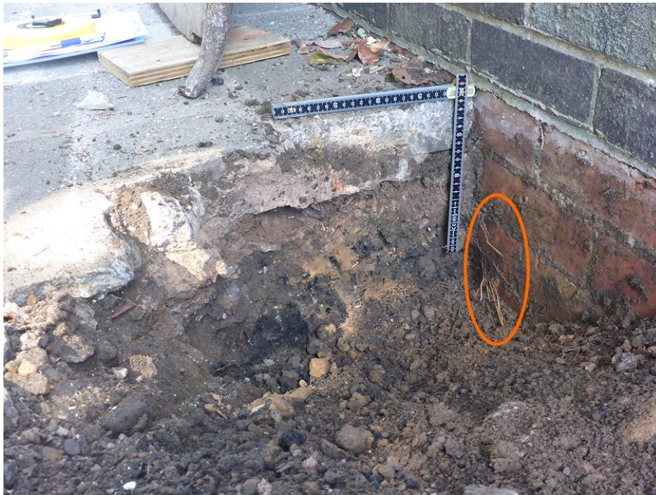
Concrete paving slabs laid on hardcore base. Fine roots found at a depth of 150mm.
