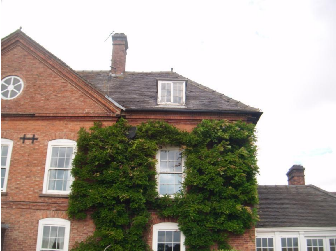
Front with decayed dormers
