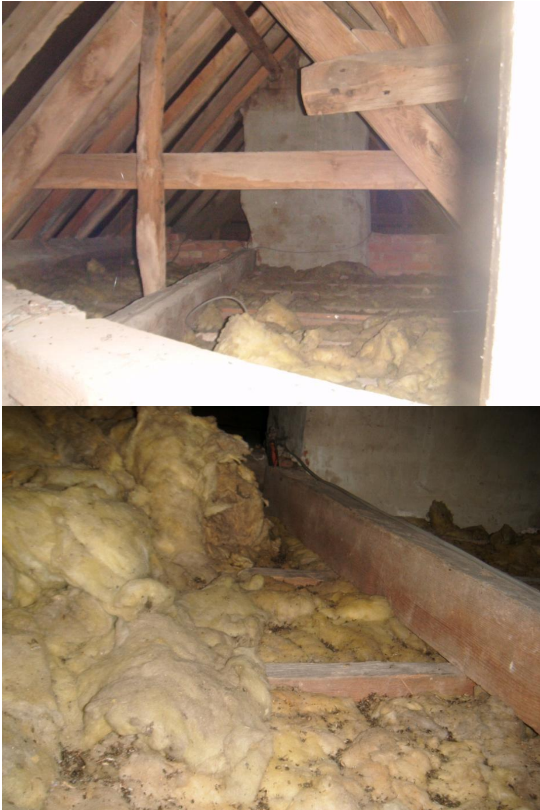
Main house loft (mainly cluster flies, some bat droppings)
