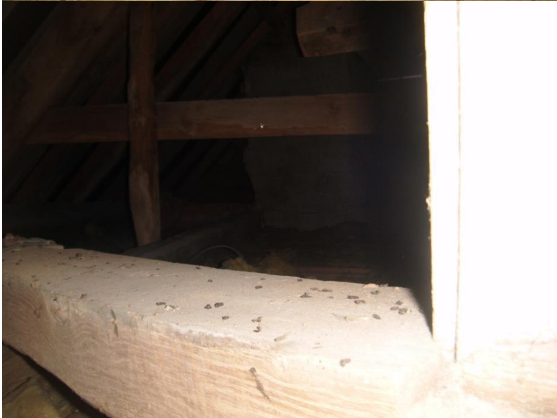
Bat droppings on beam
