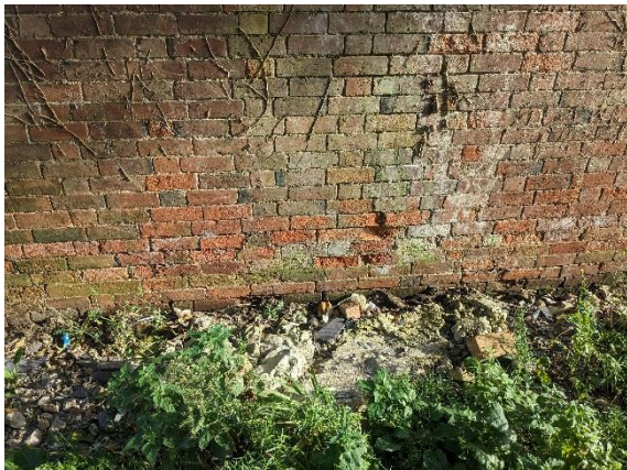
Figure 3 - Evidence of minor spalling
