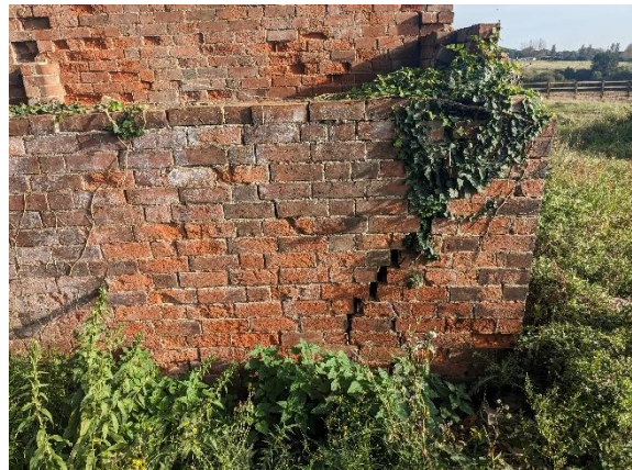
Figure 8 - Section of outbuilding wall requiring repair/localised rebuilding.
