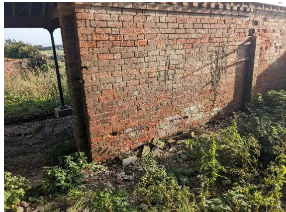
Figure 4 - Evidence of minor spalling
