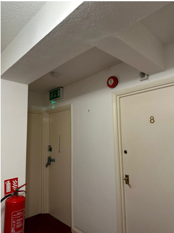
Fire mitigation measures near escape on first floor
