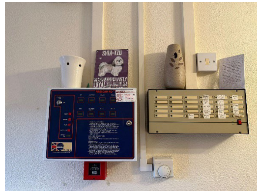
Fire Control Panel
