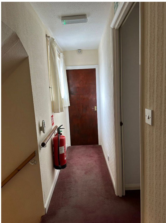
Smoke seals to fire door
