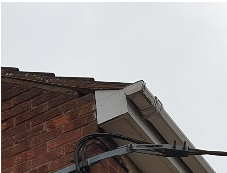
Image 4: Missing mortar at the north-eastern corner
