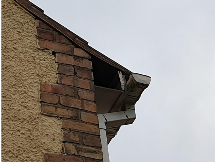
Image 3: View of missing soffit box cap
