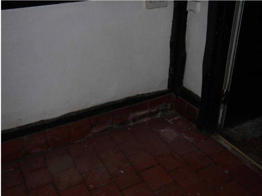
Dampness to floors. Note also rising damp to walls in original section of the building.
