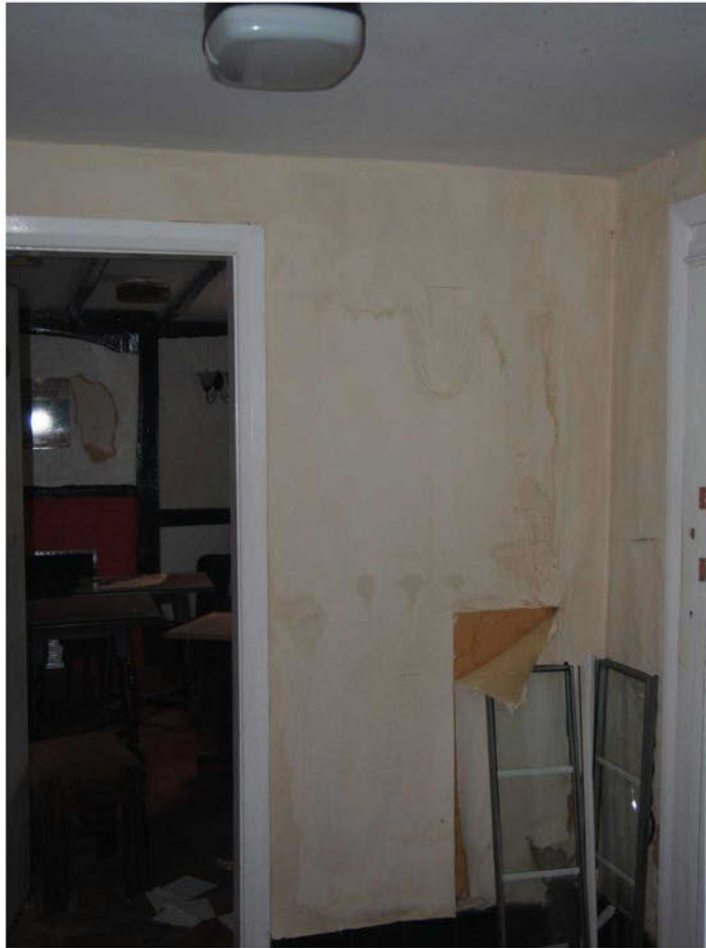
Damage to internal walls caused by dampness
