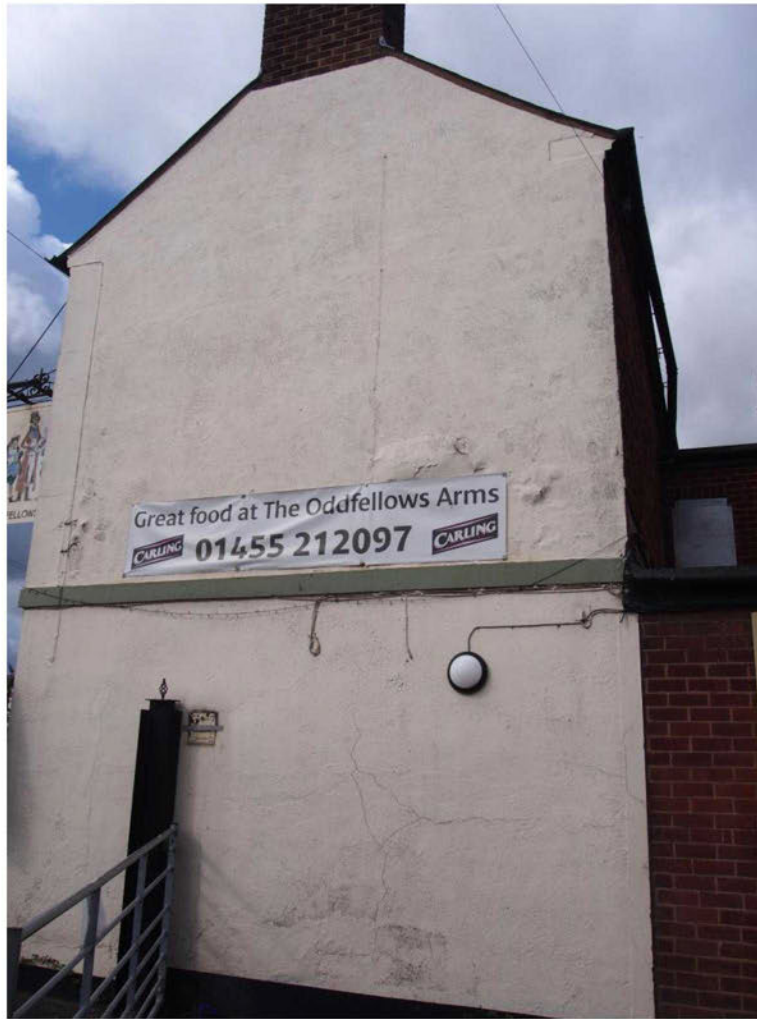
Typical poor condition of render to front and sides
