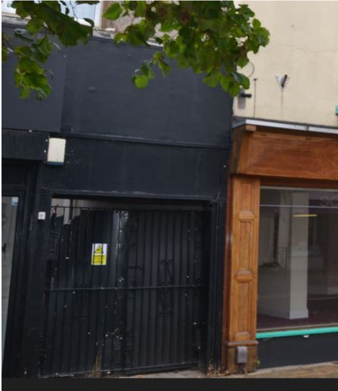
Fig. 4 Access gates to Slaughter House Yard
