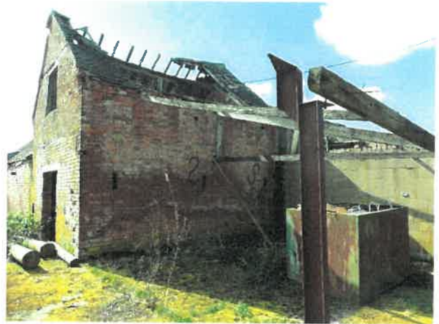
Photo 4: Collapsed roof of barn from northern elevation.
