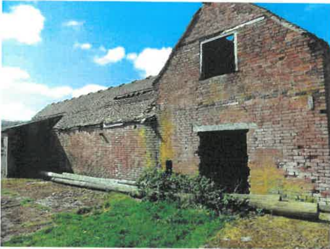
Photo 3: Open doorway and window along eastern elevation of the barn.
