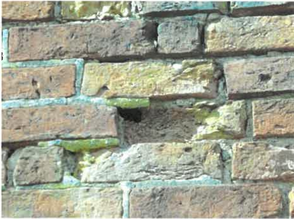
Photo 9: Crumbling brick work from western elevation.
