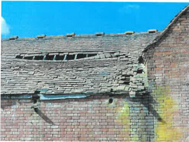
Photo 5: Missing tiles in stable 1 roof from eastern elevation.
