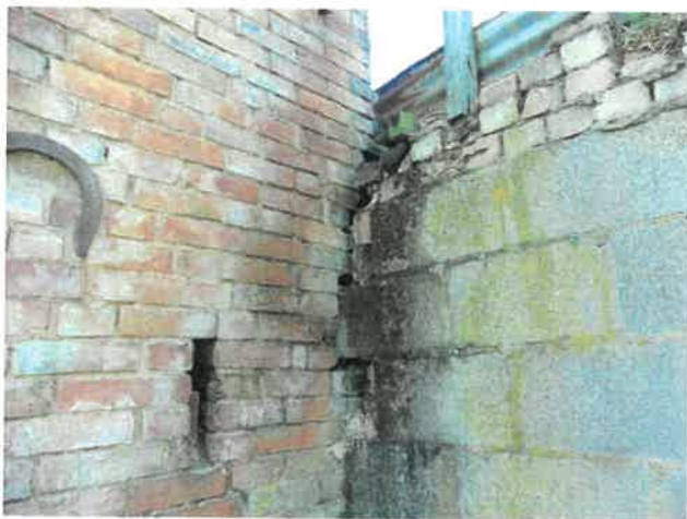
Photo 7: Cracks in brickwork between barn and adjoining cinder structure.
