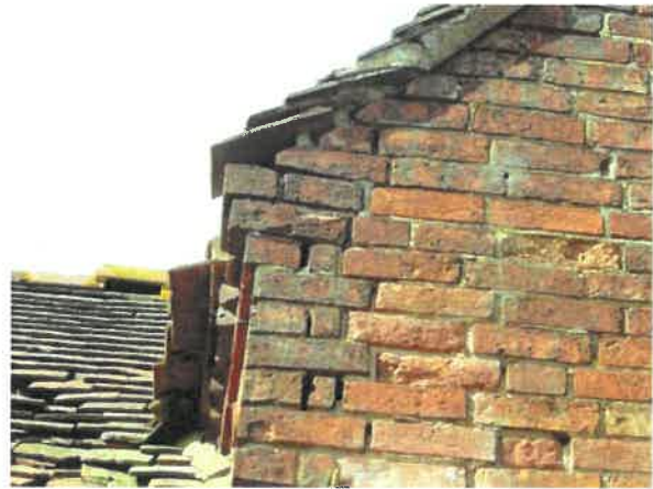
Photo 10: Missing mortar in barn roof from eastern elevation.
