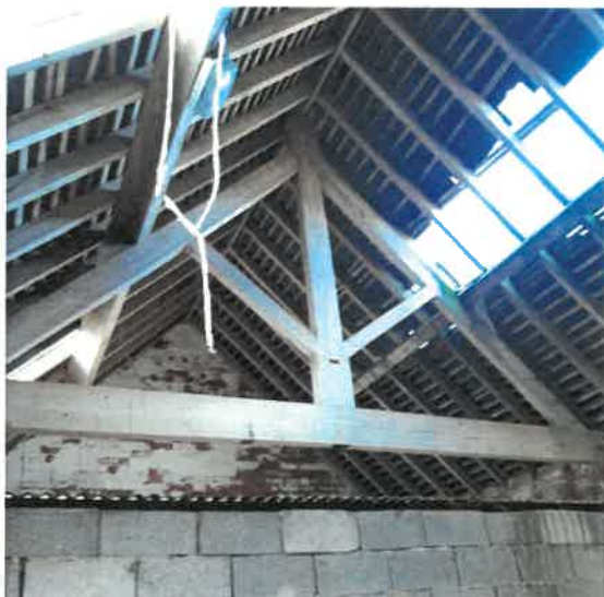
Photo 11: Open roof space created within stable block 1 and hole in roof.
