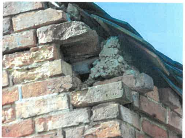
Photo 8: Crumbling brick work along barn roof.
