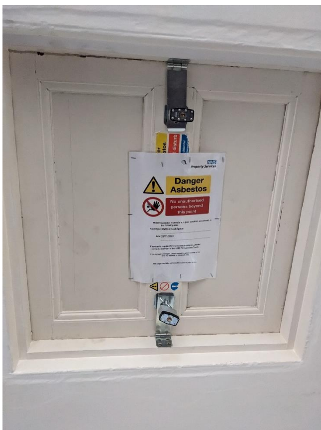
Plate 14 – Loft closed due to asbestos risk.
