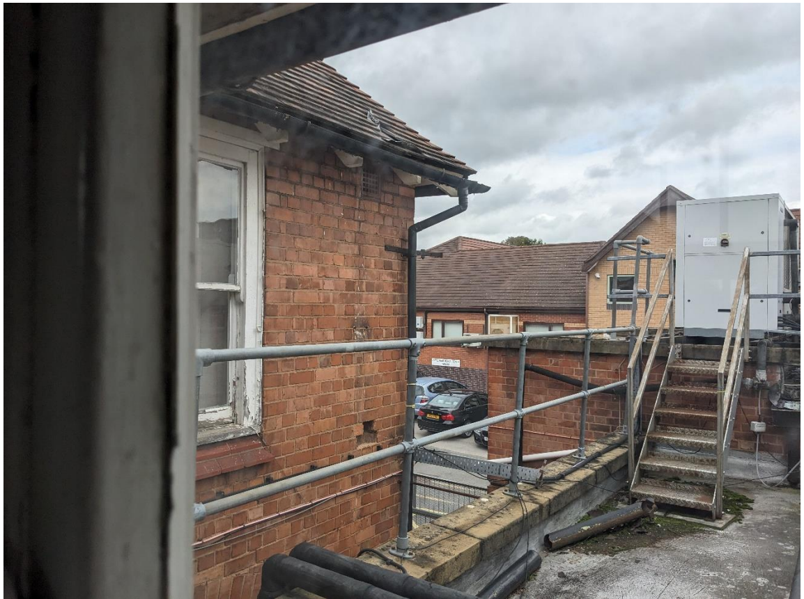
Plate 9 – Notable gaps in brickwork and disused vents.
