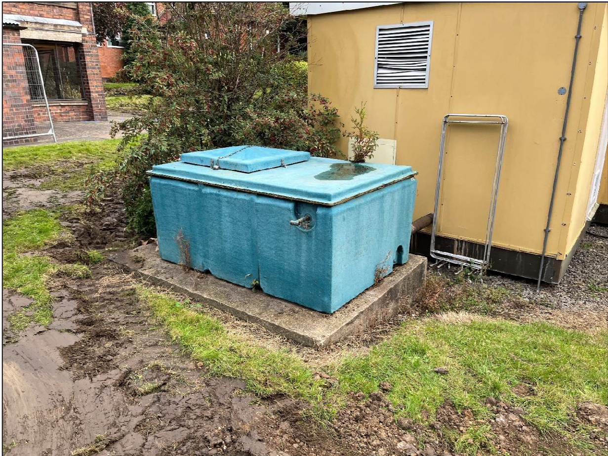
Figure 2.10-2: External tank along the north-eastern corner of the Site.
