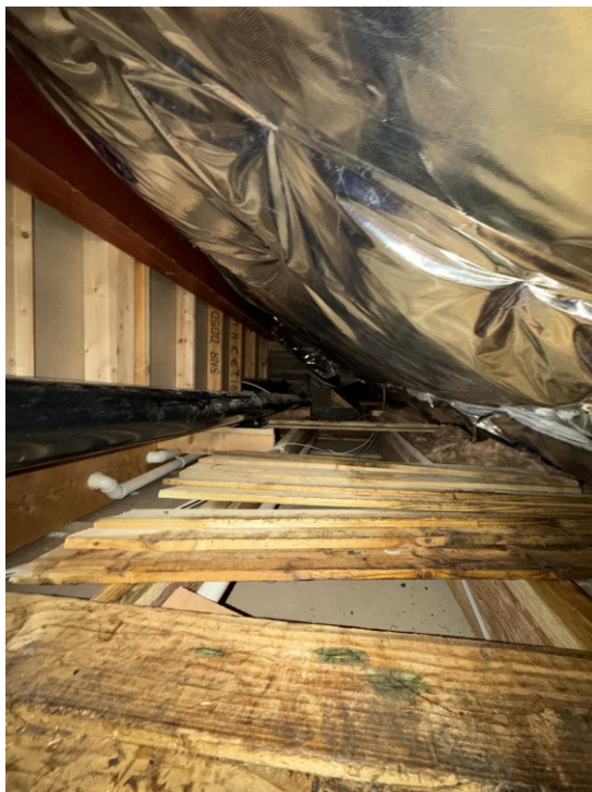
Figure 5: Roof void A in building B1
