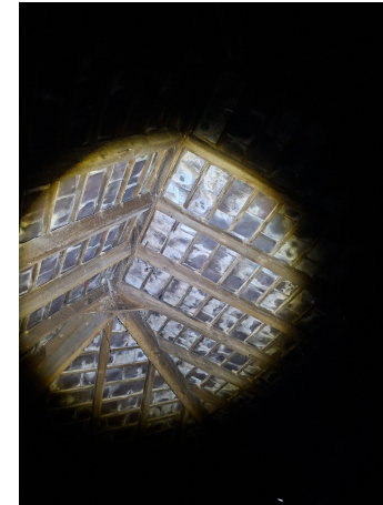
Figure 1a: Void 1 -Light ingress observed at the same areas as outlined in the PRA.
