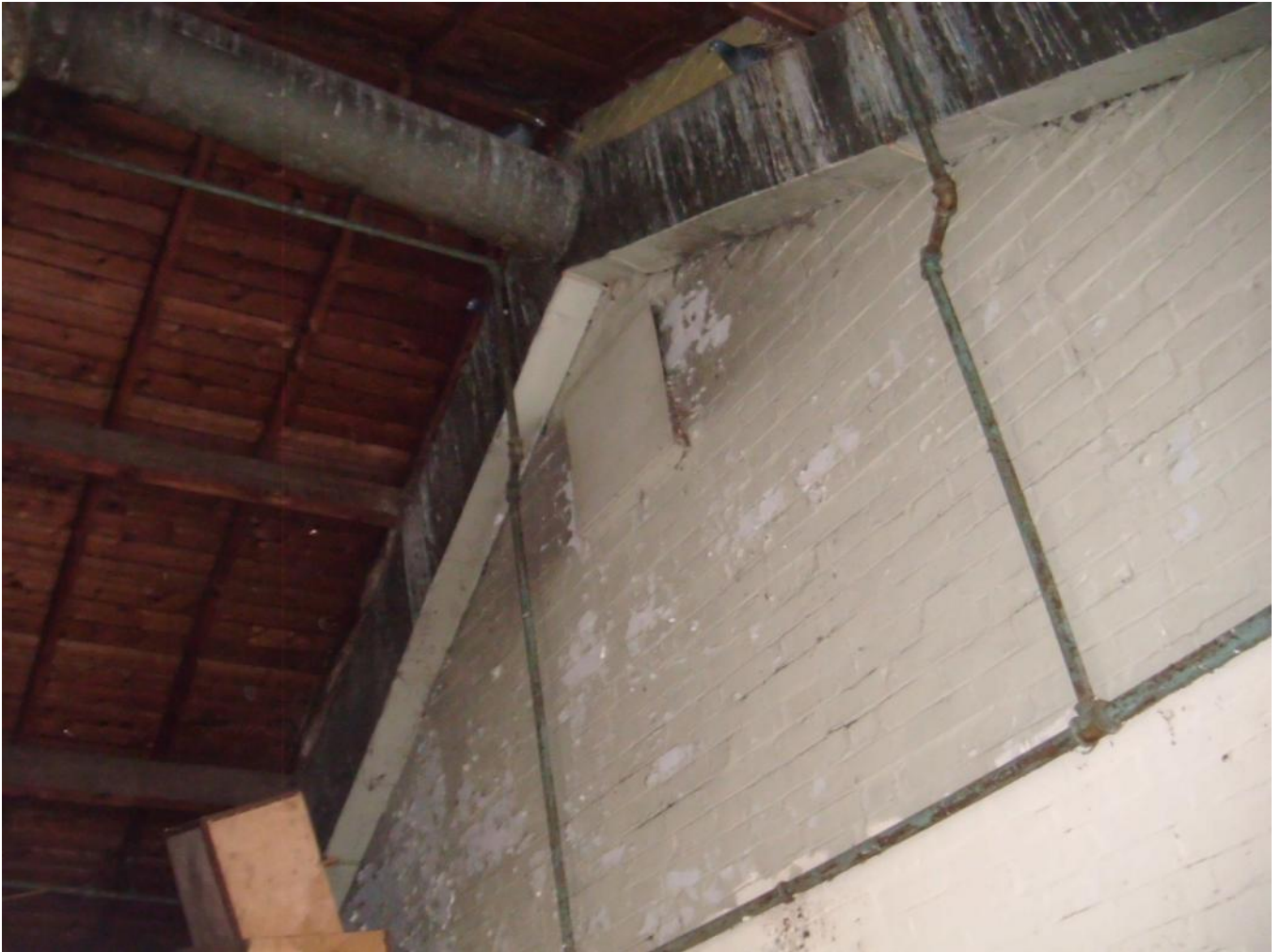
Roof lining Building 1: evidence of feral pigeon
