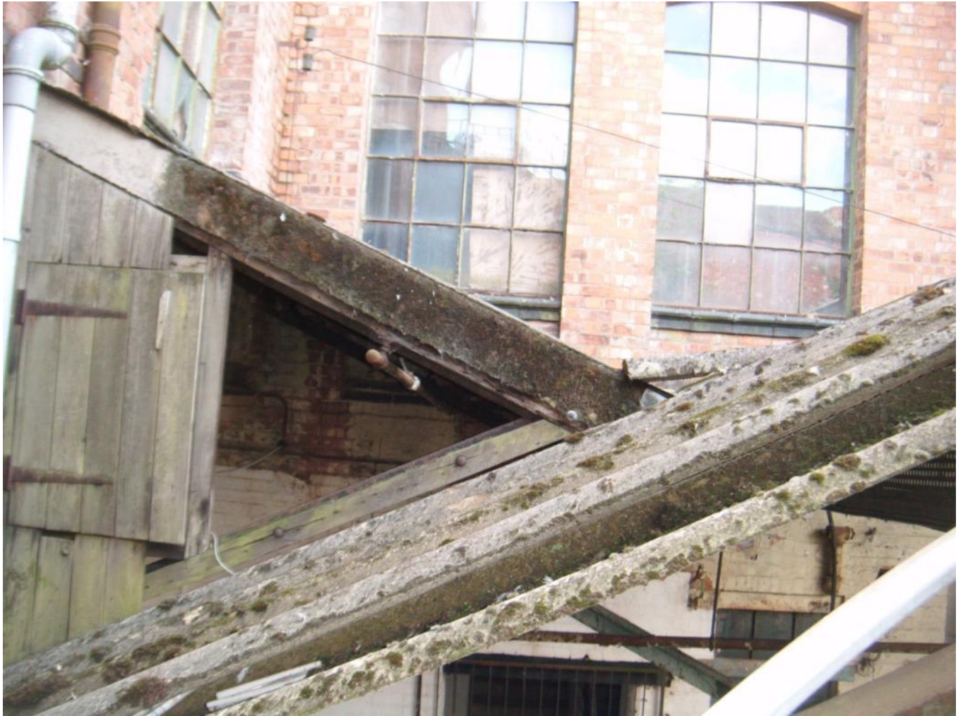
Concretious asbestos structures in courtyard
