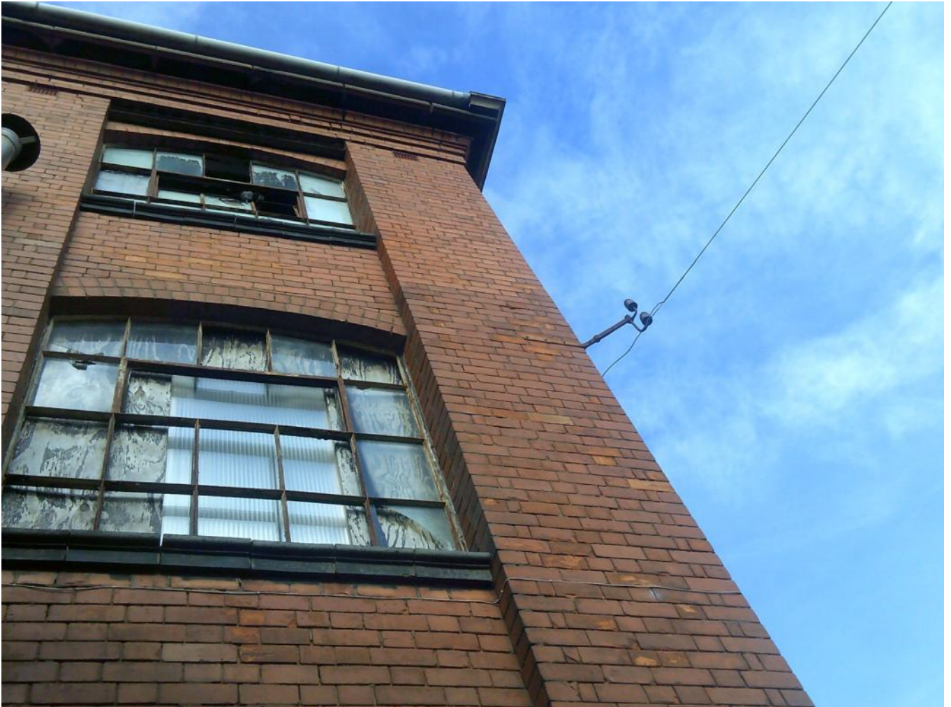
B1 (gaps are just broken windows, roof edge is corballed, no soffits)
