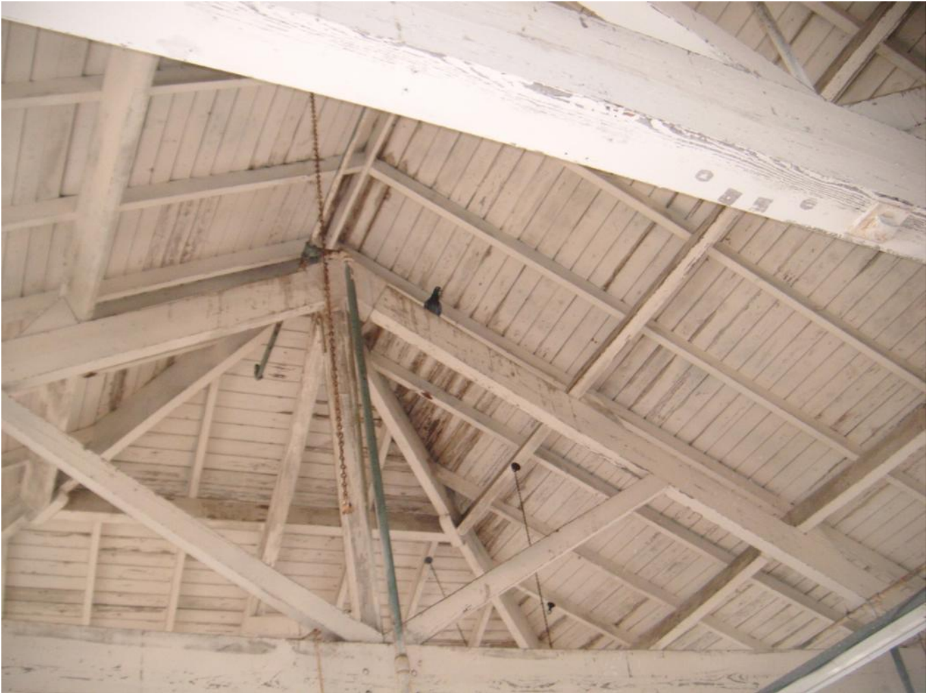
Roof lining Building 2: evidence of feral pigeon
