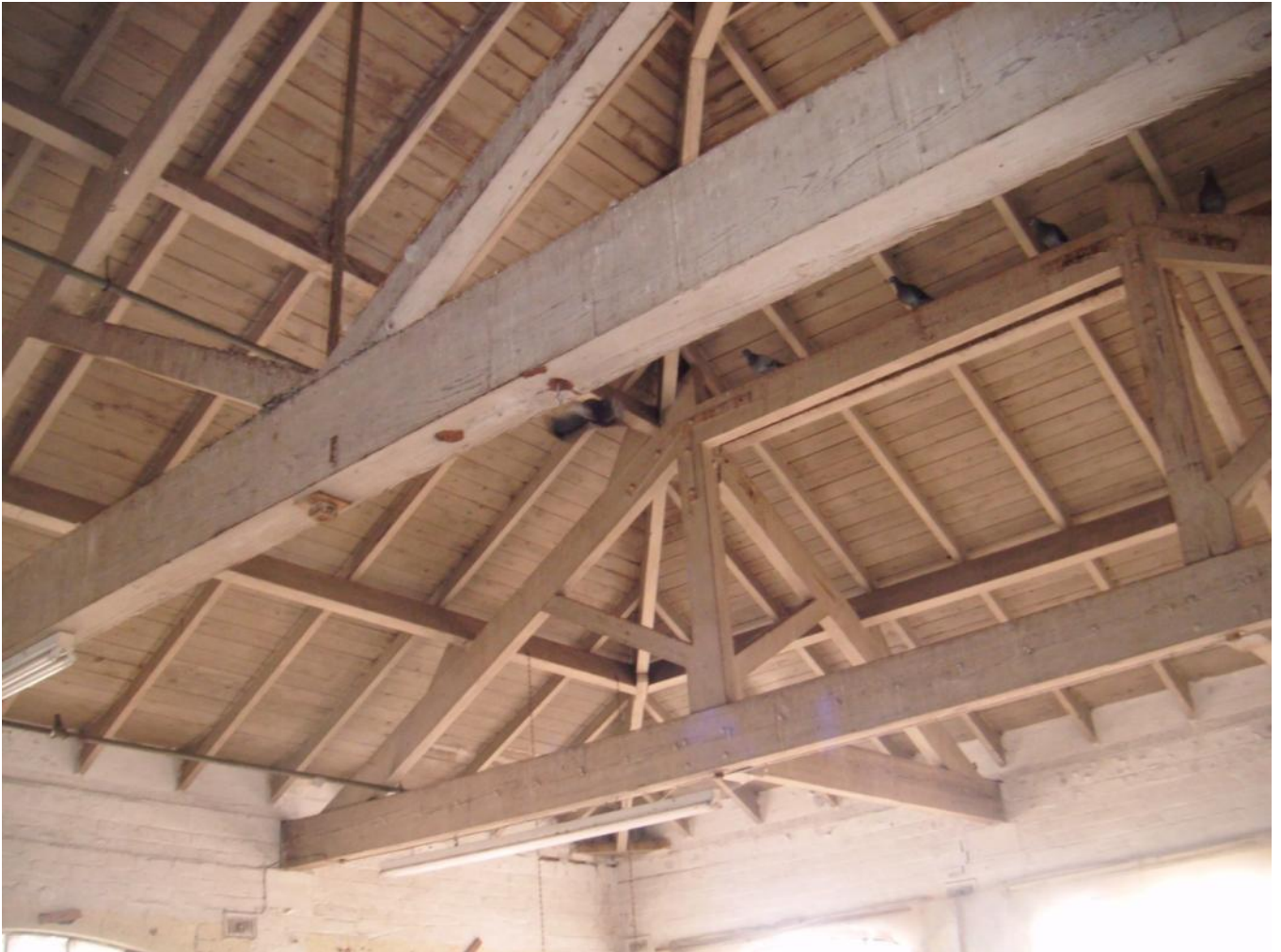
Roof lining Building 2: evidence of feral pigeon
