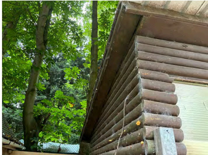
Image 10 - Condition of soffits and fascias of B2.
