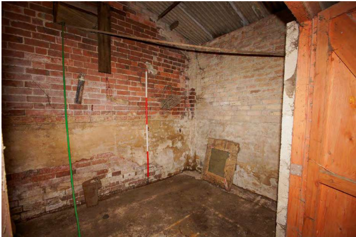
Plate 93: G8 – construction joint between the northwest and the northeast walls
