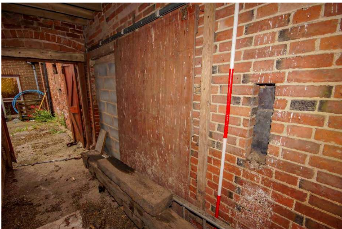
Plate 71: G3 – blocked ventilation slit
