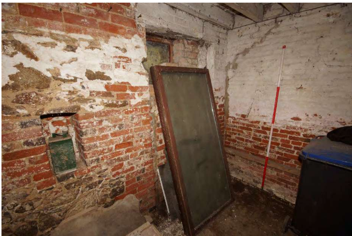
Plate 60: G1 – detail of blocked ventilation slit and doorway
