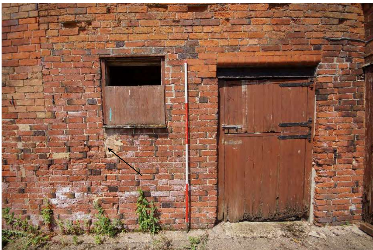
Plate 10: Building 1 – southeast elevation, detail of construction joint and blocked ventilation slit (arrow)
