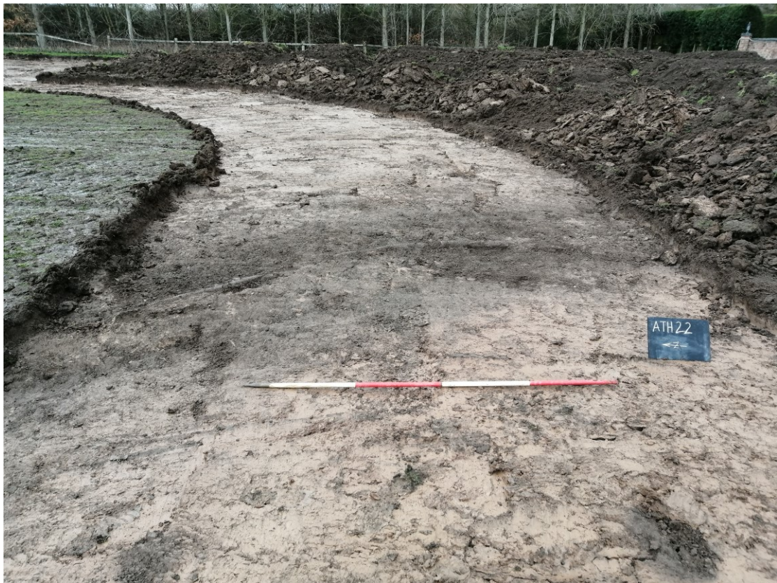
Plate 7; electric cable in new access road, view east.
