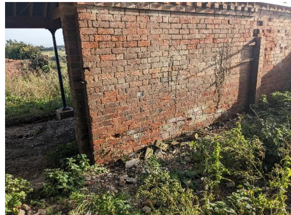
Figure 4 - Evidence of minor spalling
