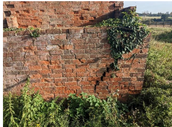
Figure 8 - Section of outbuilding wall requiring repair/localised rebuilding.
