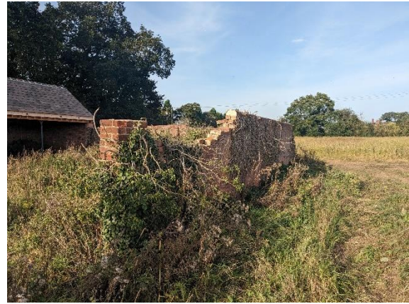
Figure 10- Are of courtyard wall that requires repair/localised rebuilding.
