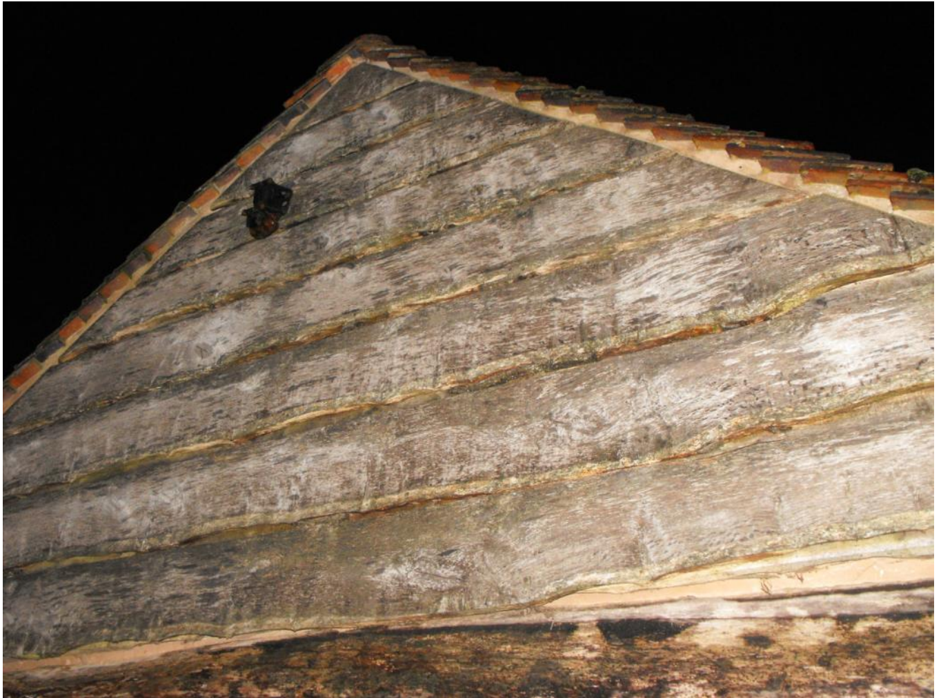
External tight fitting oak boarding
