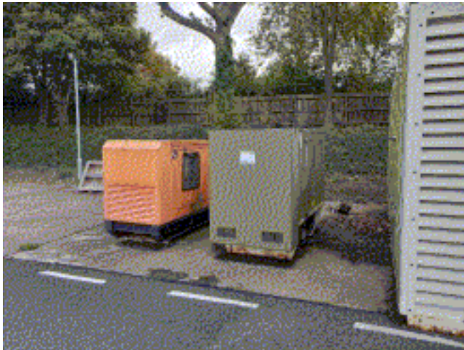
Photo 7: Electricity generators located adjacent to the eastern site boundary. The slope to the adjacent land is shown in the background of the picture.
