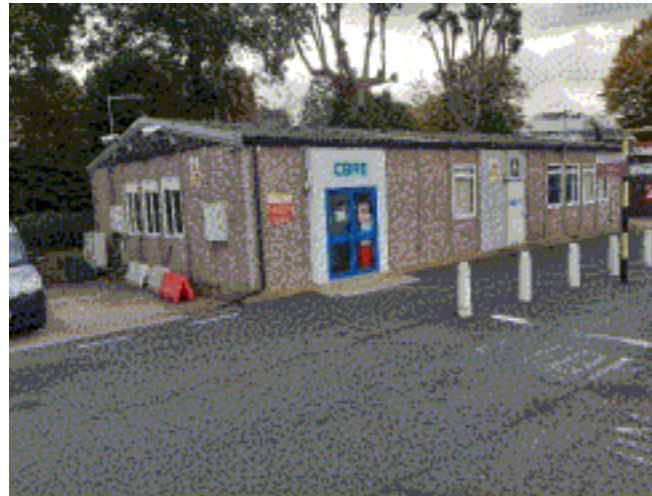
Photo 8: Building in the south-eastern corner with suspected asbestos roofing.
