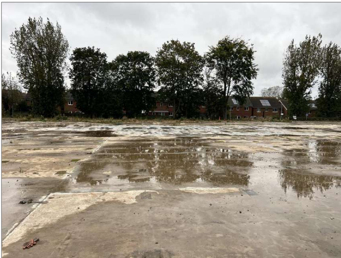
Photo 13. Example of hardstanding
