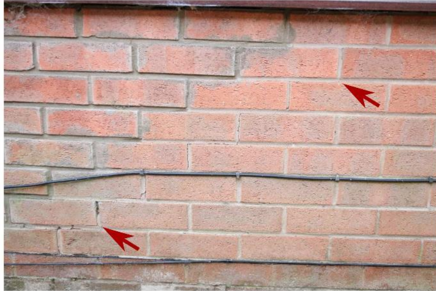
Damage - Current Damage
