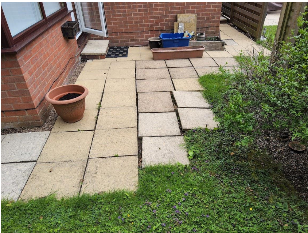
Photo 5 – Uneven garden paving
