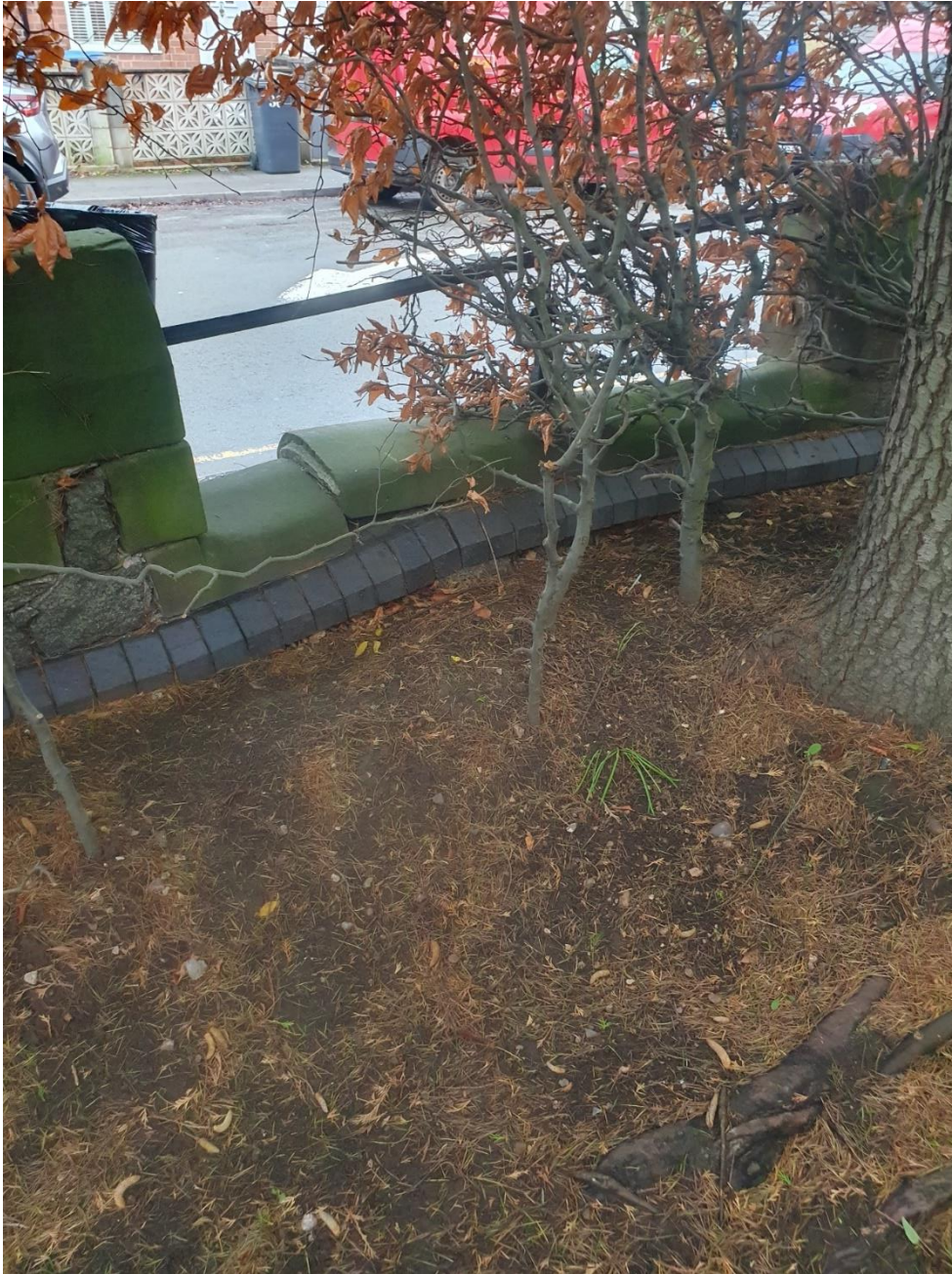
Tree B roots are pushing up the stone wall and damaging it.
