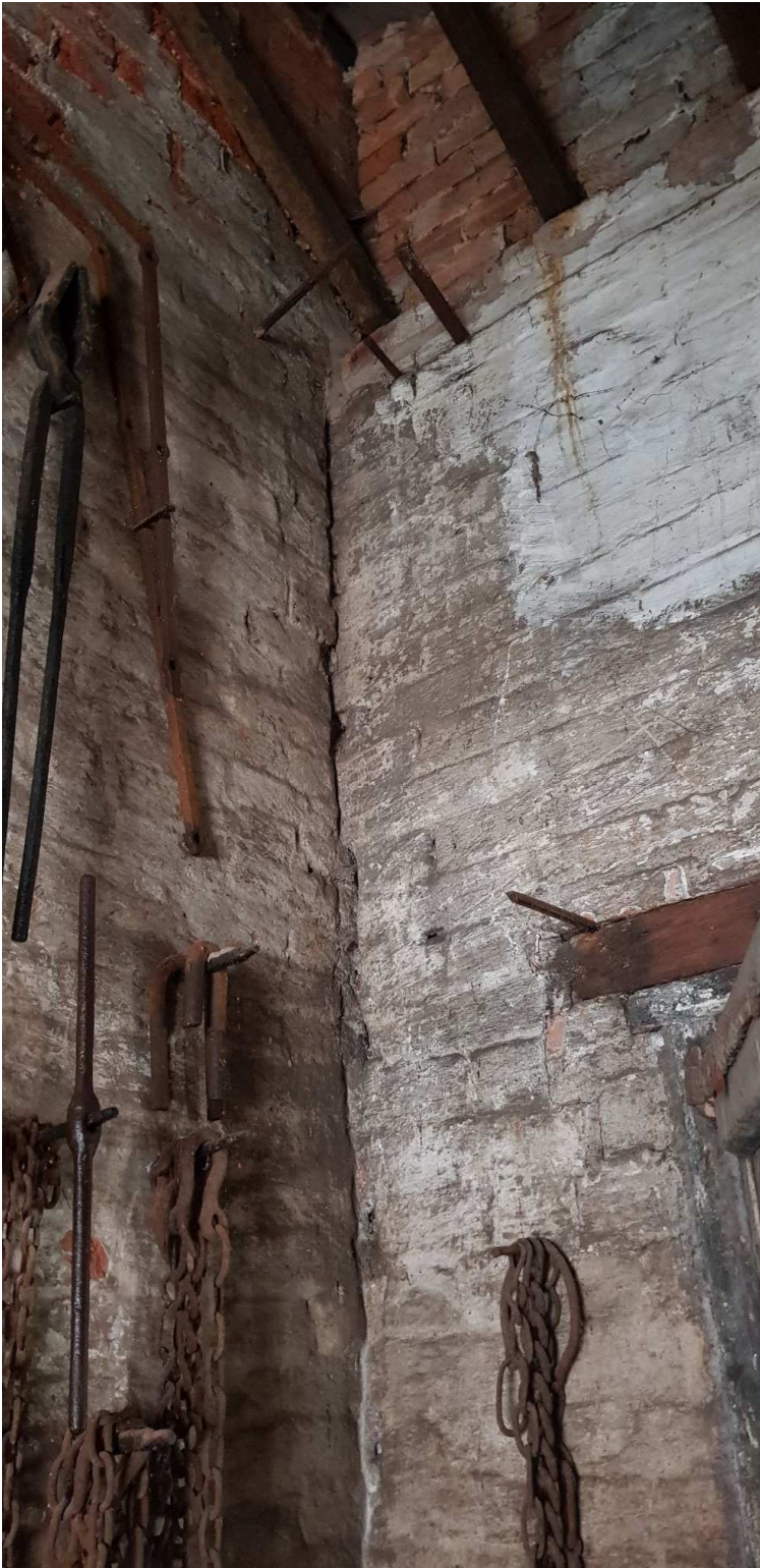
Photo 23 Old Forge Large Crack in Masonry to Internal Corner
