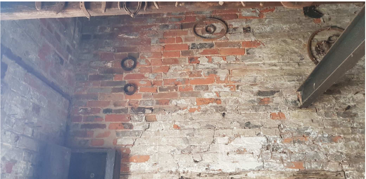
Photo 20 Old Forge Poor Brickwork Generally
