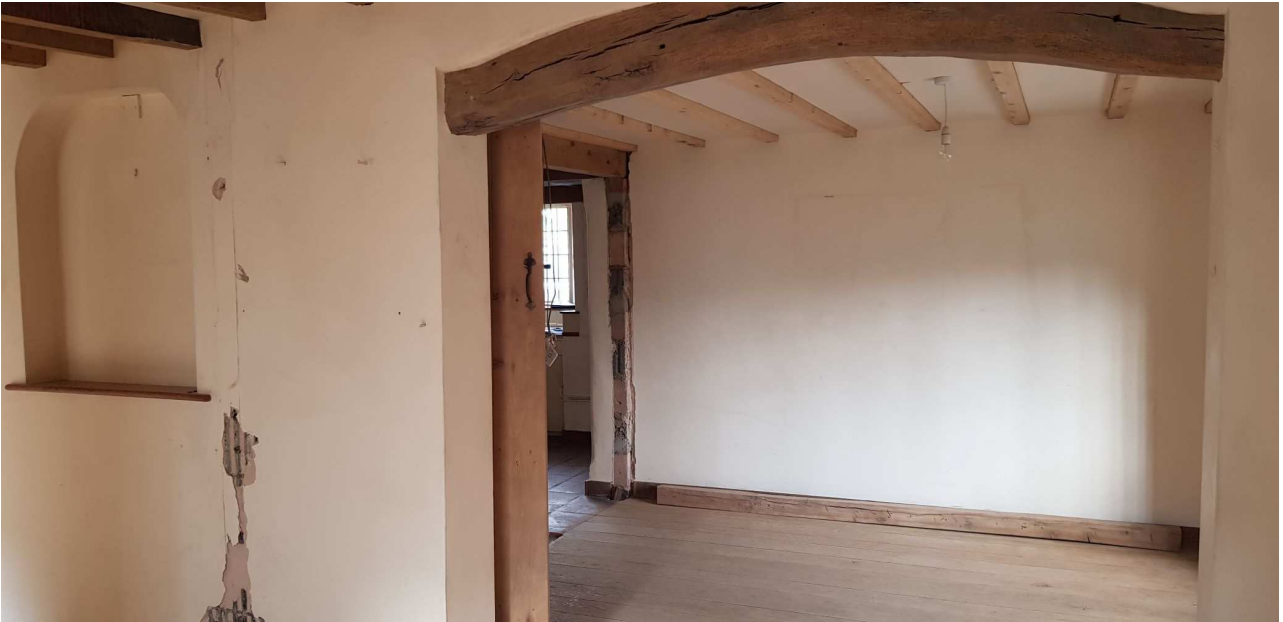
Photo 9 Split Timber Beam in Kitchen
