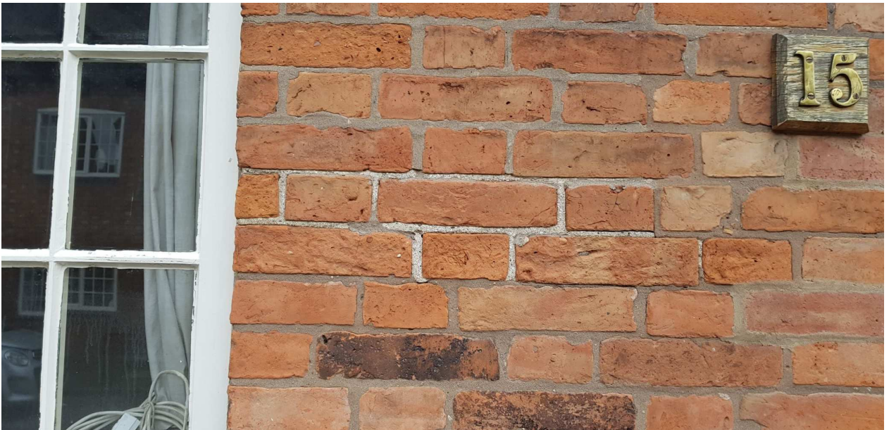
Photo 32 Previous Repointing carried out with Sand/Cement Mortar over Lime Based Mortar
