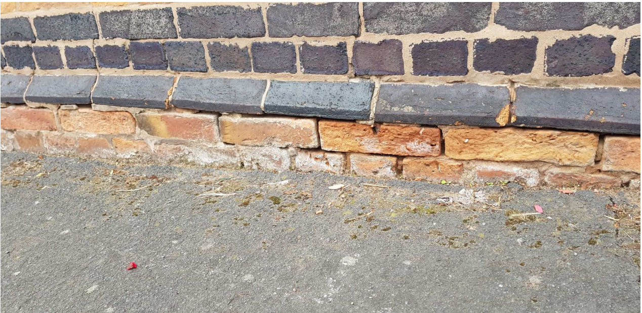
Photo 34 Poor Condition Masonry and Mortar Below DPC Level to Front Wall
