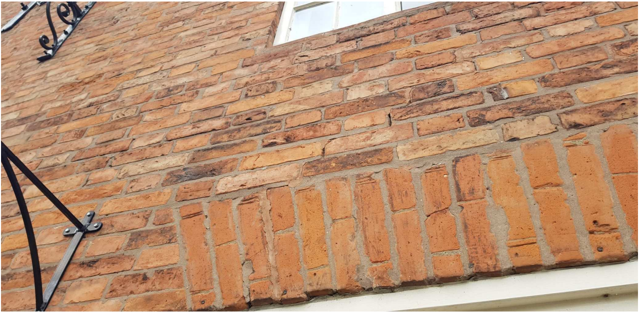
Photo 31 Movement in Masonry Over Front Windows
