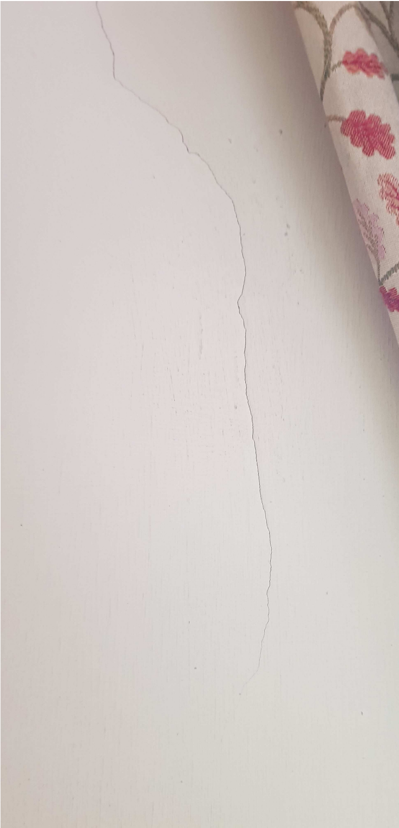
Photo 15 First Floor Minor Cracks in Wall
