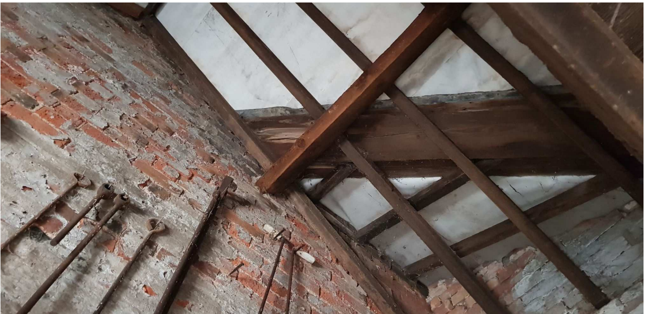
Photo 22 Old Forge Poor Brickwork to End Wall
