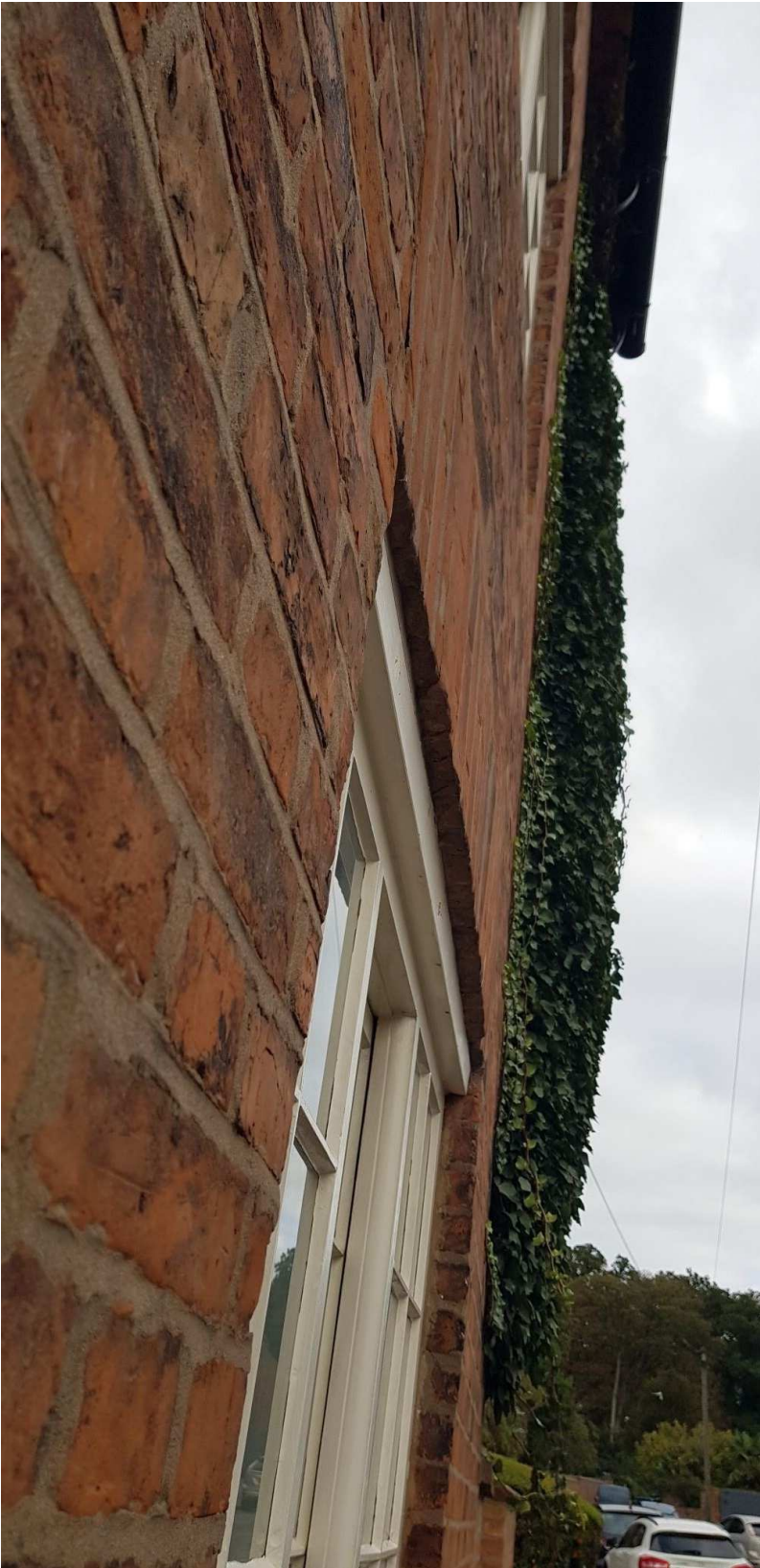
Photo 30 Bulging Masonry to Soldier Course Over Front Windows
