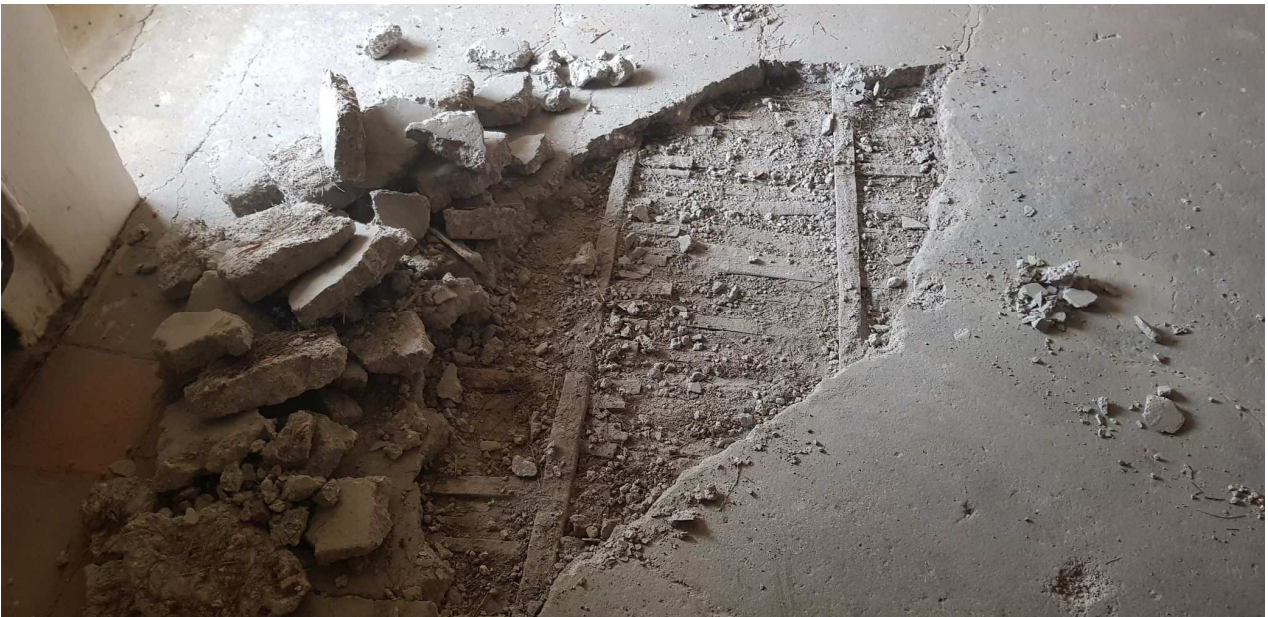
Photo 17 Damage to Floor-Note Unusual Concrete Topping
