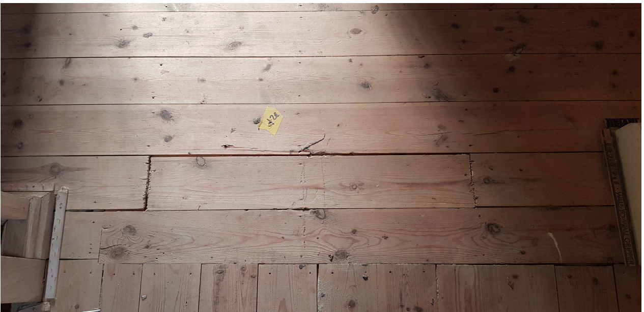
Photo 14 First Floor Opening of Floor Board Joints
