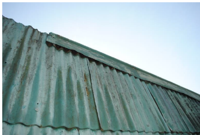
B1 – area of flashing
