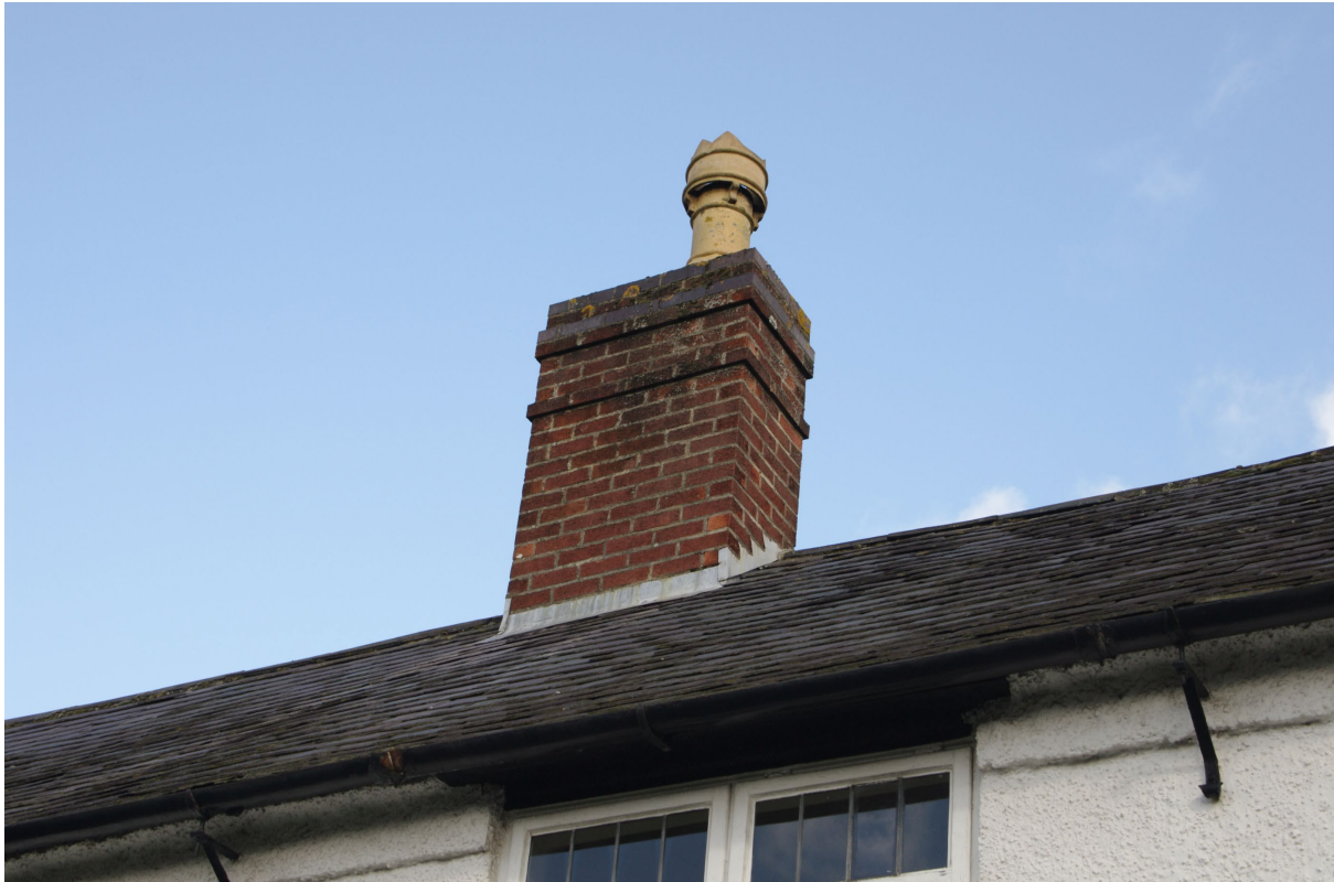
Figure 16: Central chimney stack seen from SW elevation Only one pot belonging to No 37 remains despite being a double flue stack
