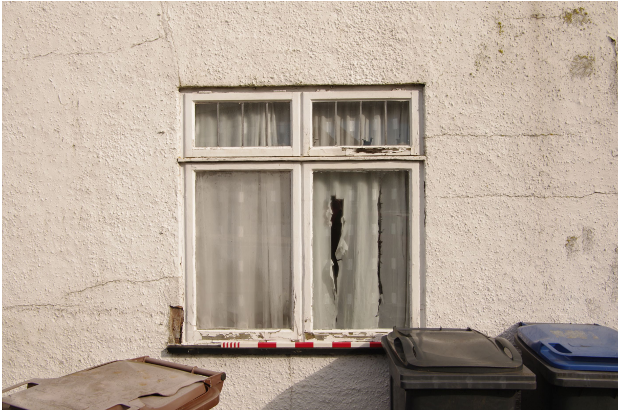
Figure 18: SW facing elevation of No 37, ground floor window detail to left of door Looking north-east. 1m scale. Note the parallel cracks in the render which may point to joints, or possible timberwork, within the wall structure
