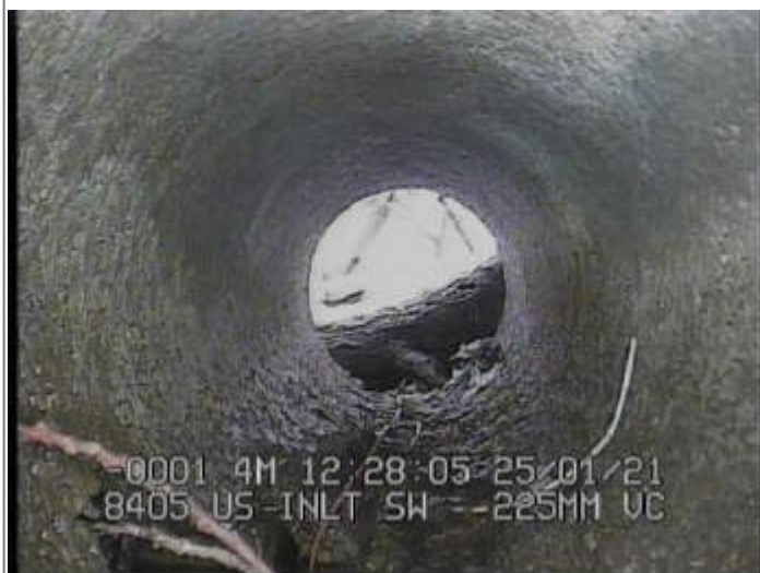
Hole in drain/sewer from 5 to 8 o'clock
