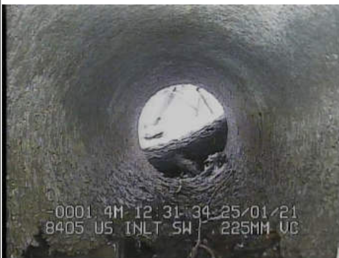
Survey Abandoned - Remark: HOLE UNABLE TO PASS
