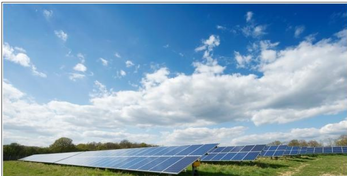
Figure 4.1: A Typical Operational Solar Farm
