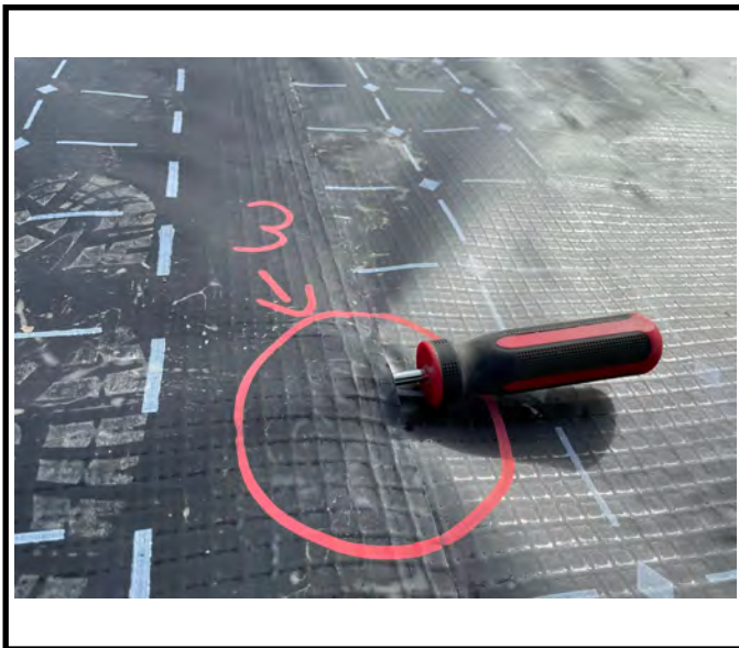
A fault identified.
