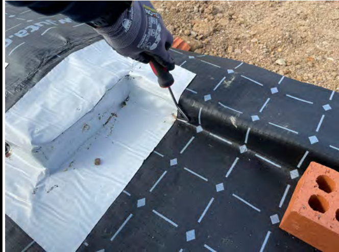
A mechanical point stress test being conducted upon a sealed corner.
