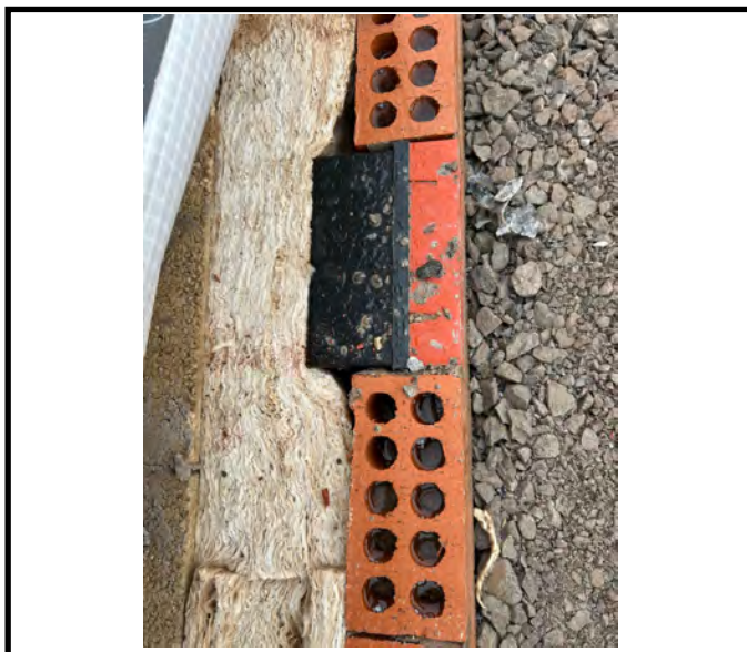
An overview of a periscopic vent connecting to an air brick.
