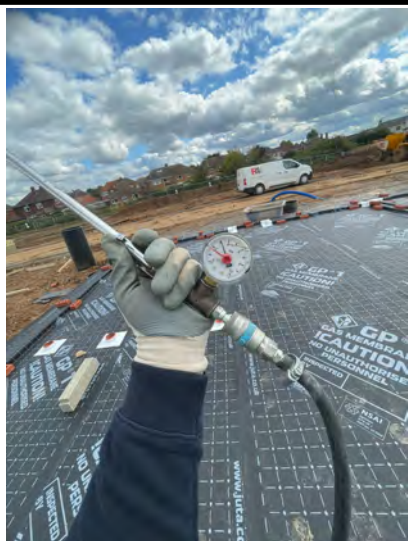
Correct pressure achieved.
