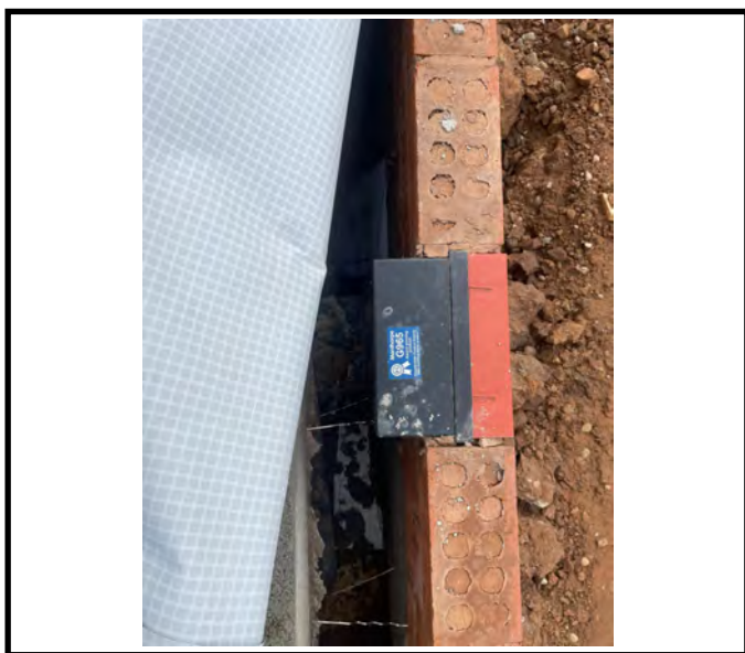
An overview of the telescopic vent connected to the air brick.
