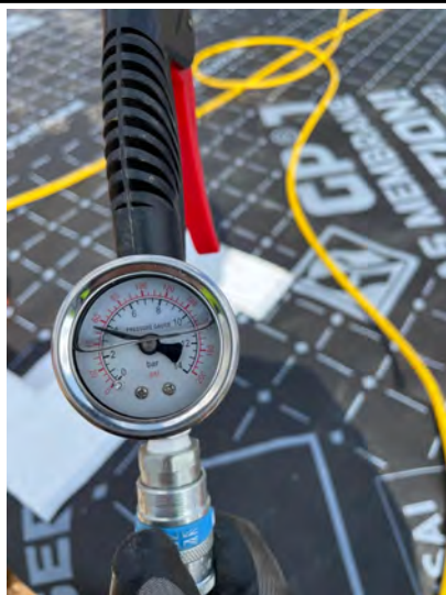
Correct pressure achieved.
