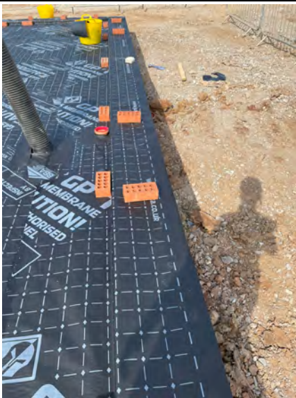
An overview of sealed pipe penetrations.
