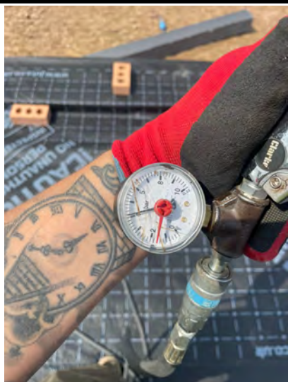
Correct pressure achieved.
