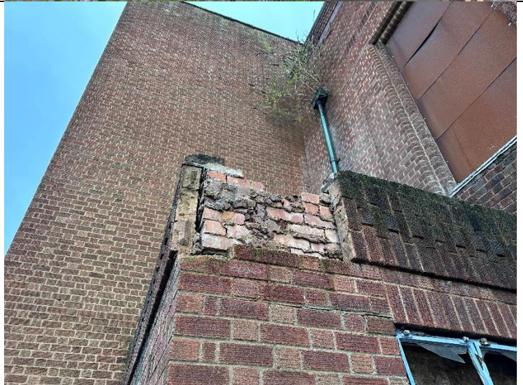
Image 6: Image showing small opening in brickwork on eastern aspect of the building.
