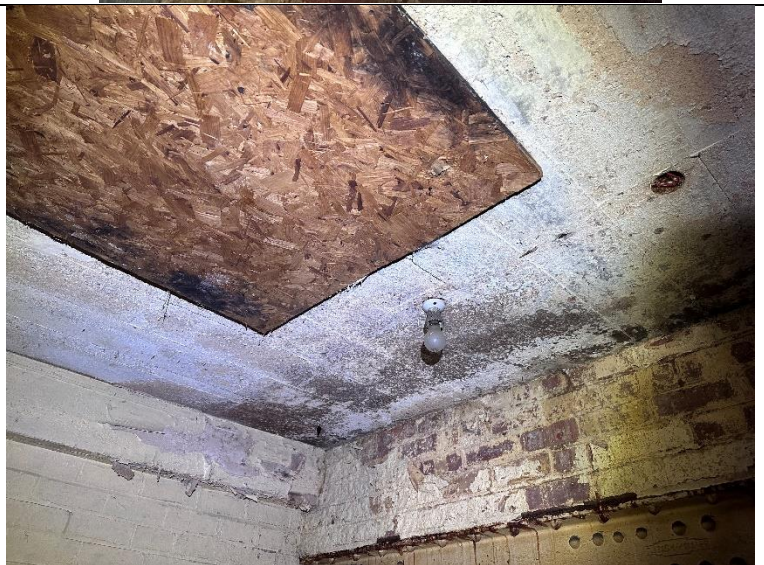
Image 12: Image showing condition of typical flat roofed section of the building.
