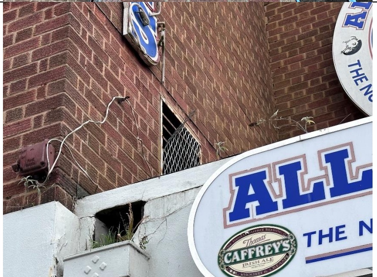
Image 7: Image showing indicative open vent on northern aspect of the building.
