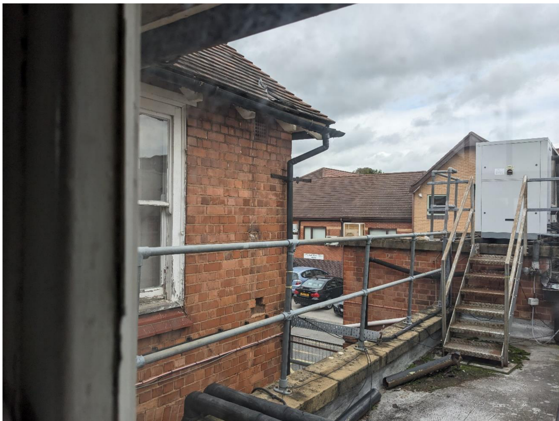
Plate 9 – Notable gaps in brickwork and disused vents.
