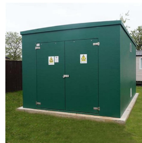
Sub Station Example
