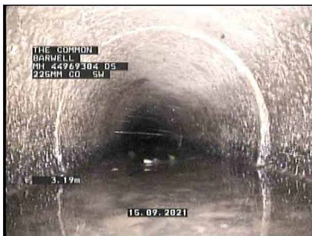
44969304X_c8b9277b-d51e-4de4-a6bf-7dcb52b176a3_202109 15_092856_250.jpg, 00:02:38, 3.10 m Settled deposits, other, 30% cross-sectional area loss, start, Stones
