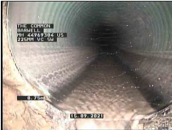
_X_af490d8f-1502-4e2d-b38c-858b3ffb67ac_20210915_09210 0_473.jpg, 00:00:22, 0.70 m Material changes to asbestos cement
