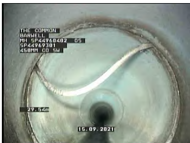
SP44968402X_213e87f8-b81c-473a-867b-c9baa1e2c6bd_20210915_114137_685.jpg, 00:03:28, 29.50m Other obstacles in invert from 10 o'clock to 2 o'clock, 5% cross-sectional area loss, joint seal
