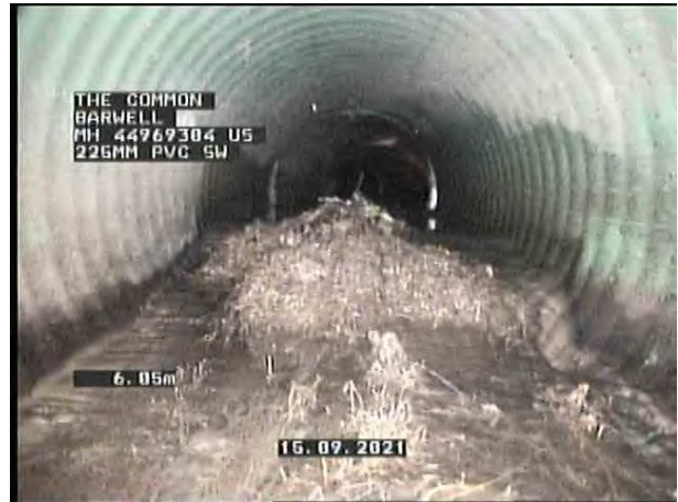
_X_5f304ae7-a971-4180-bdd8-d945b1fa45b4_20210915_0922 46_352.jpg, 00:01:37, 6.00 m Roots, mass, 60% cross-sectional area loss
