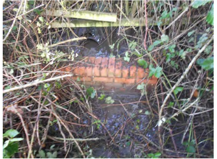
END OF FIELD DITCH AT IFHW3 NOTE FIELD DITCH SILTED U/S OF HW & D/S OF HW HIGHWAY DRAINAGE DITCH
