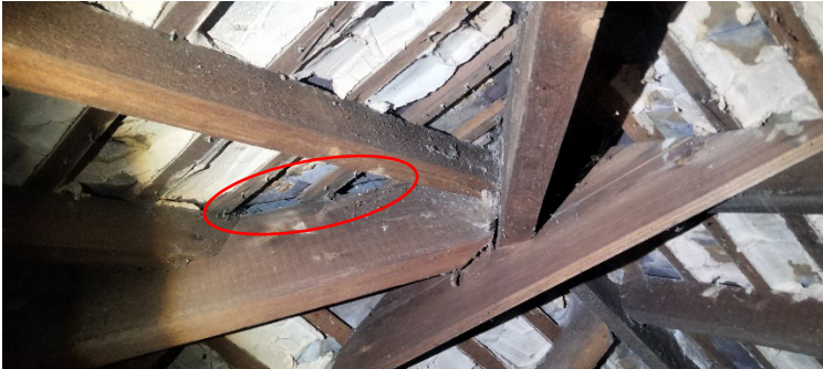
Figure 14. Light ingress (gap under hip tile) on the southwestern hip line
