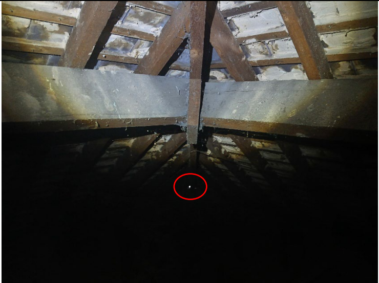
Figure 13. Light ingress (gap at end hip tile) within B1 loft space
