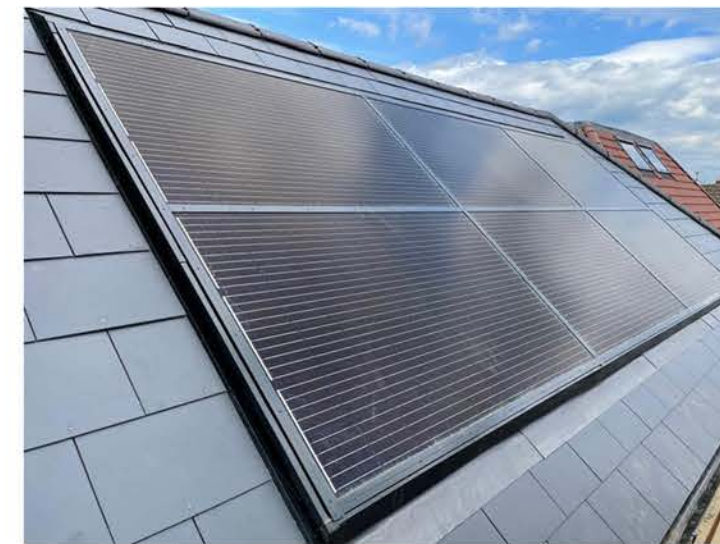
Solar Panels (roof mounted)
