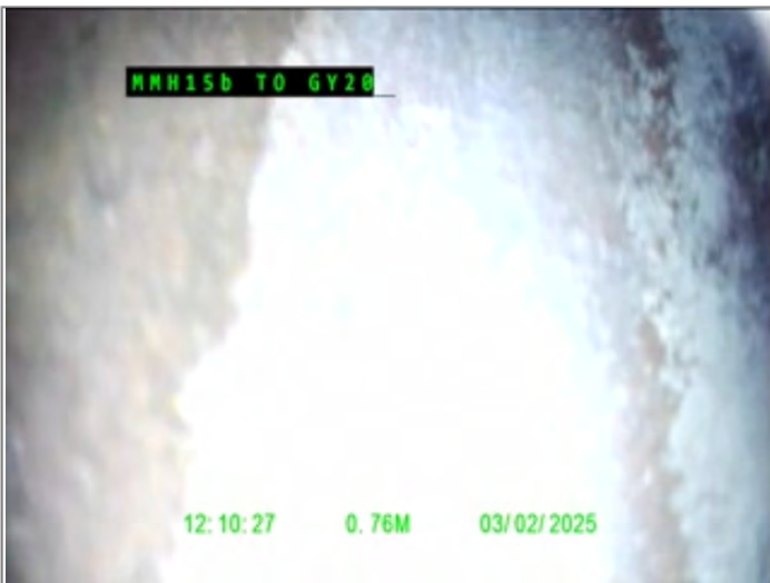
Line of drain/sewer deviates up
