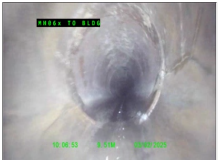
Crack longitudinal at 3 o'clock at joint
