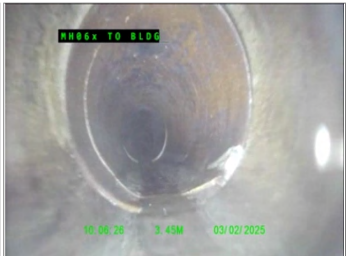
Crack circumferential from 4 to 11 o'clock at joint
