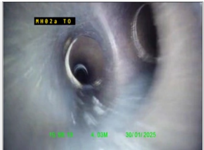
Connection other than junction at 3 o'clock, diameter 150mm
