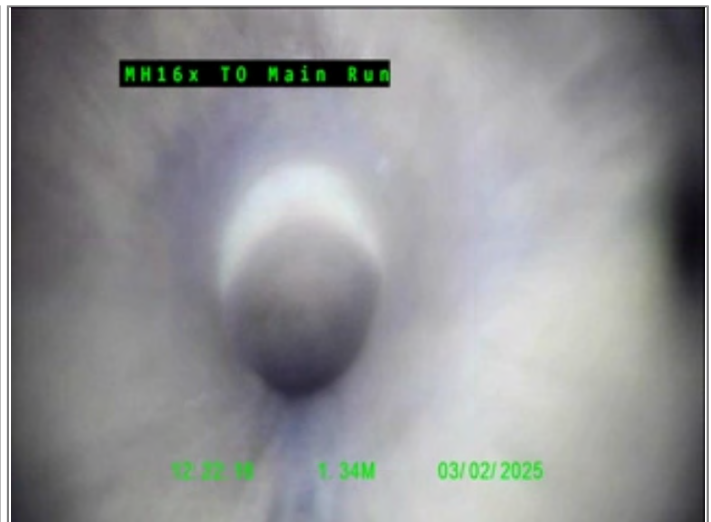
Joint displaced 10mm
