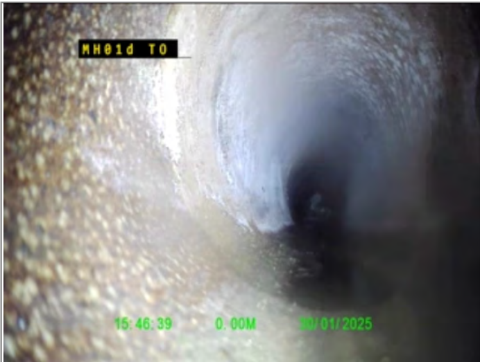
Start node type, Manhole, reference MH01d
