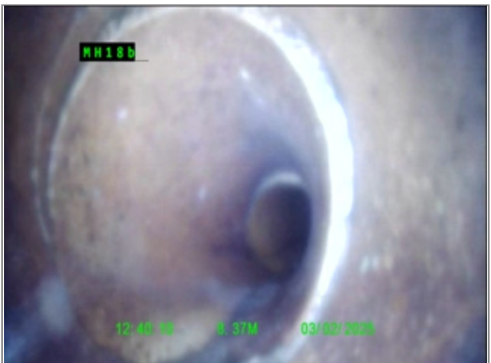
Line of drain/sewer deviates right
