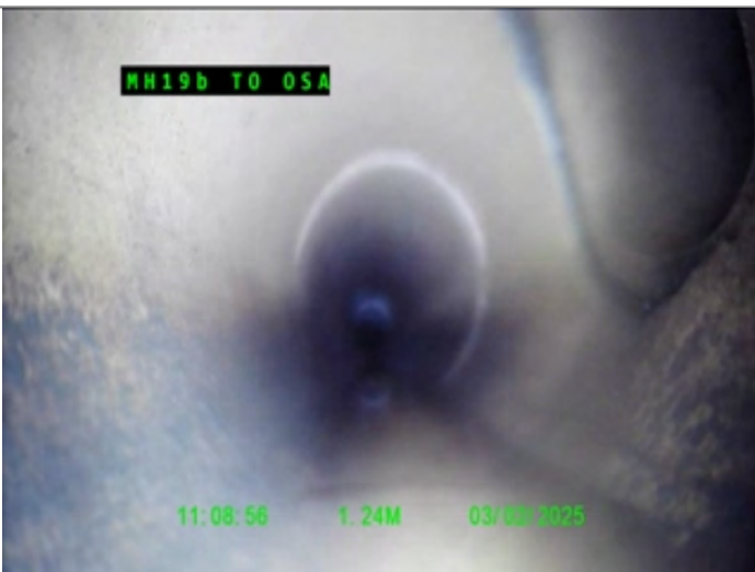
Connection other than junction at 2 o'clock, diameter 100mm
