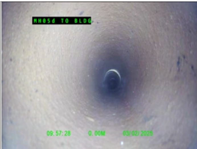
Start node type, Manhole, reference MH05d
