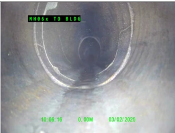
Crack circumferential from 3 to 10 o'clock at joint
