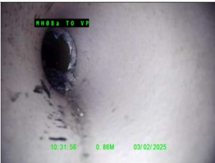
Line of drain/sewer deviates left
