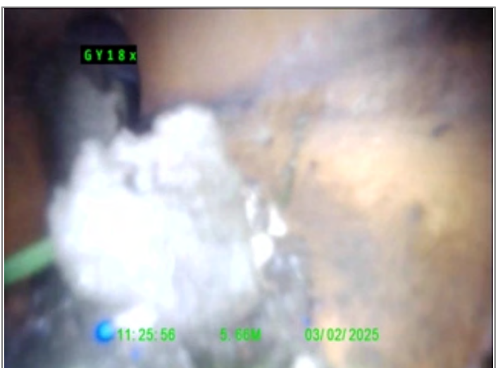
Line of drain/sewer deviates left
