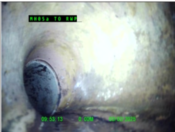
Line of drain/sewer deviates left
