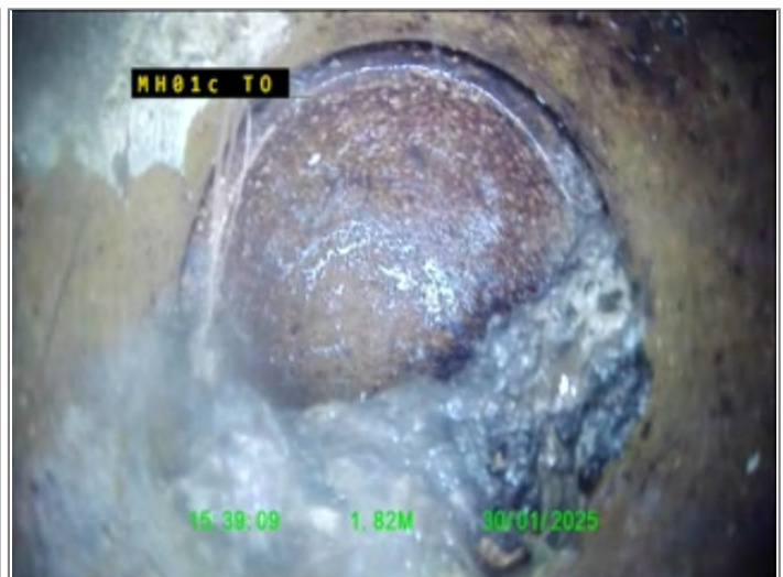
Settled deposits fine 20% cross-sectional area loss
