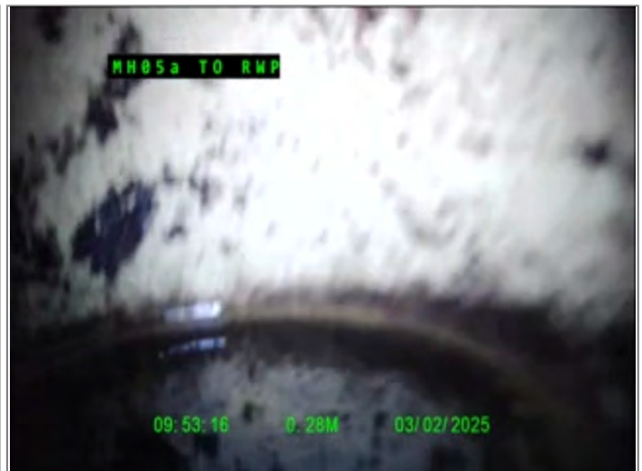
Line of drain/sewer deviates down
