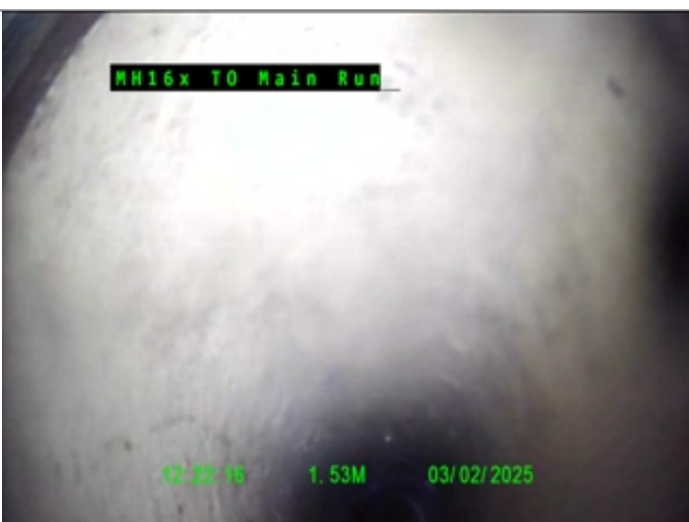
Line of drain/sewer deviates down
