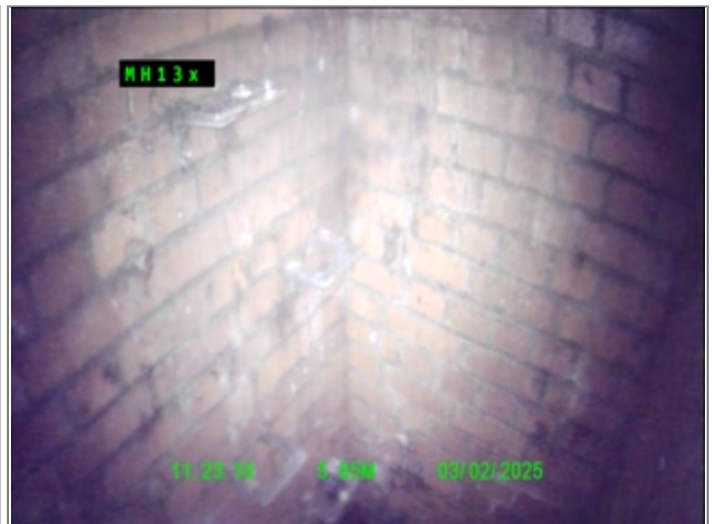
Finish node type, manhole, reference MH OSA
