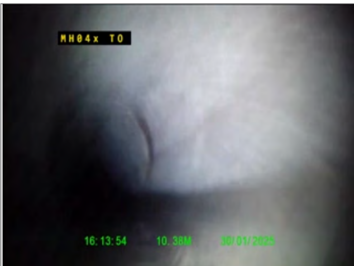
Line of drain/sewer deviates left
