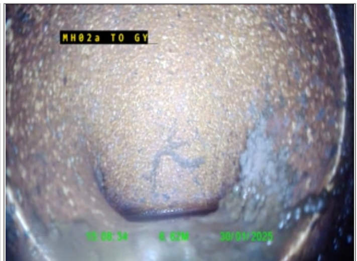
Line of drain/sewer deviates down
