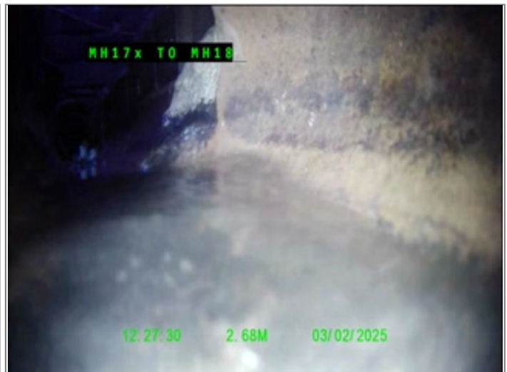
Line of drain/sewer deviates left
