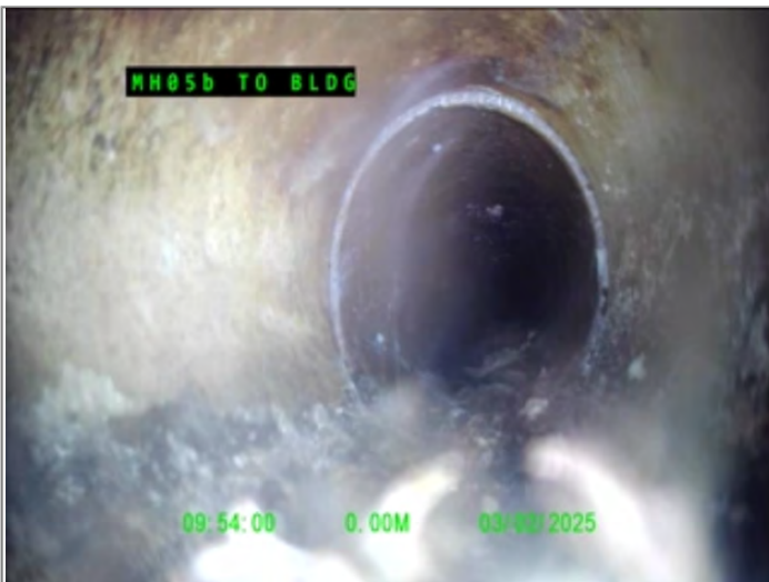
Settled deposits fine 5% cross-sectional area loss, Start
