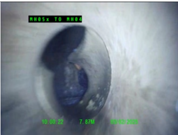
Line of drain/sewer deviates left
