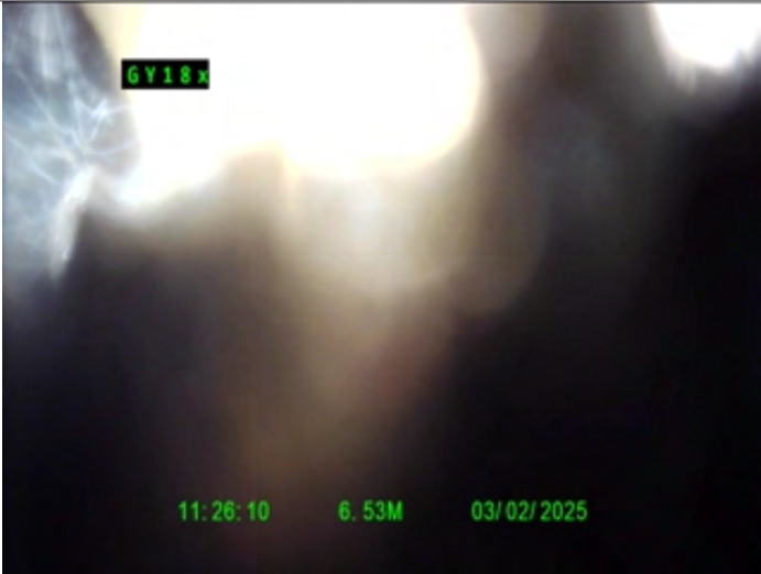
Loss of vision, silt
