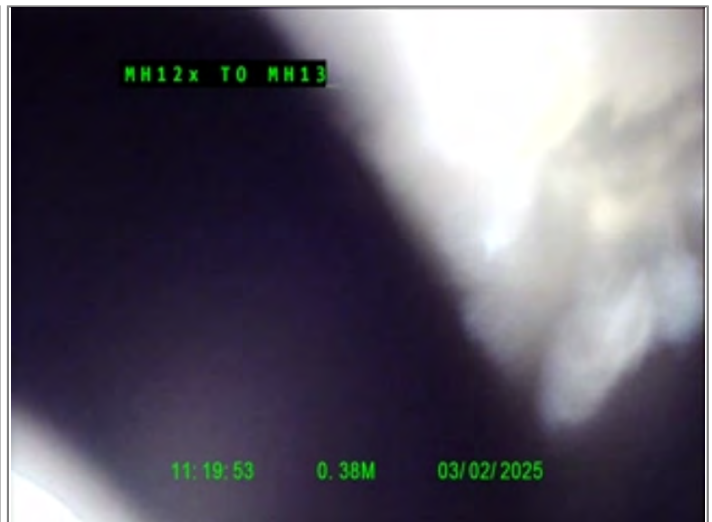
Loss of vision, silt
