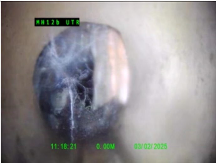
Settled deposits coarse 10% cross-sectional area loss
