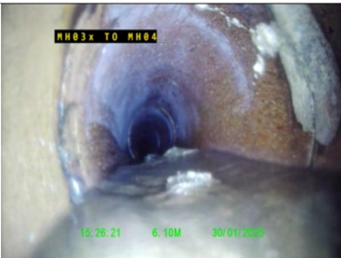
Settled deposits fine 10% cross-sectional area loss
