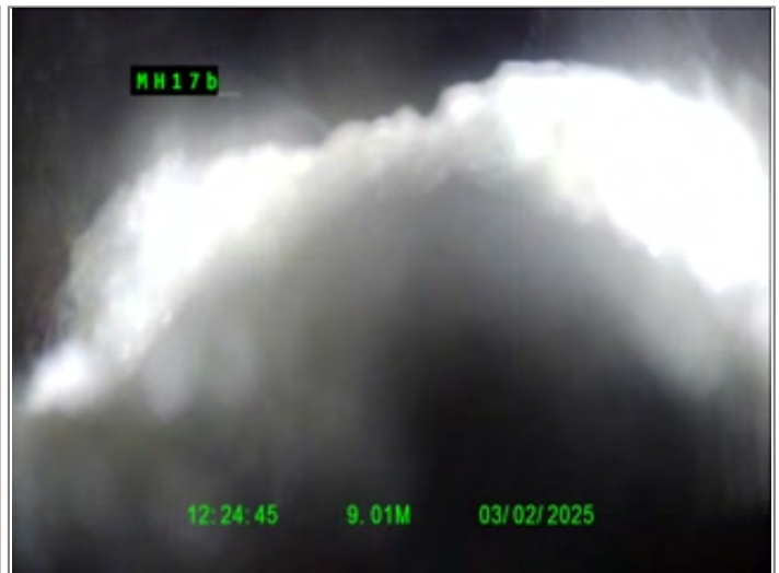
Settled deposits fine 30% cross-sectional area loss
