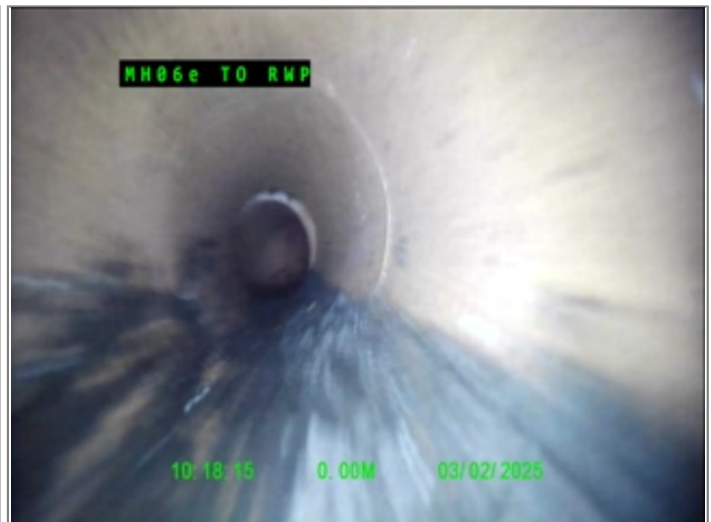
Crack circumferential from 1 to 5 o'clock
