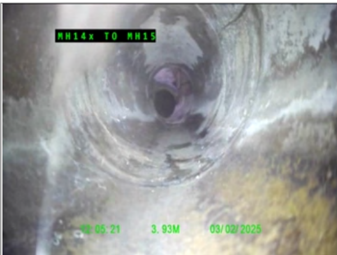
Crack longitudinal at 2 o'clock at joint
