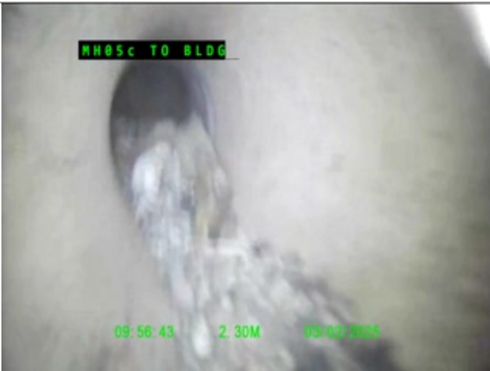
Line of drain/sewer deviates left
