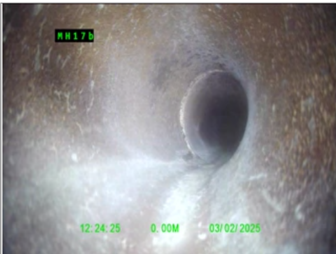
Line of drain/sewer deviates right
