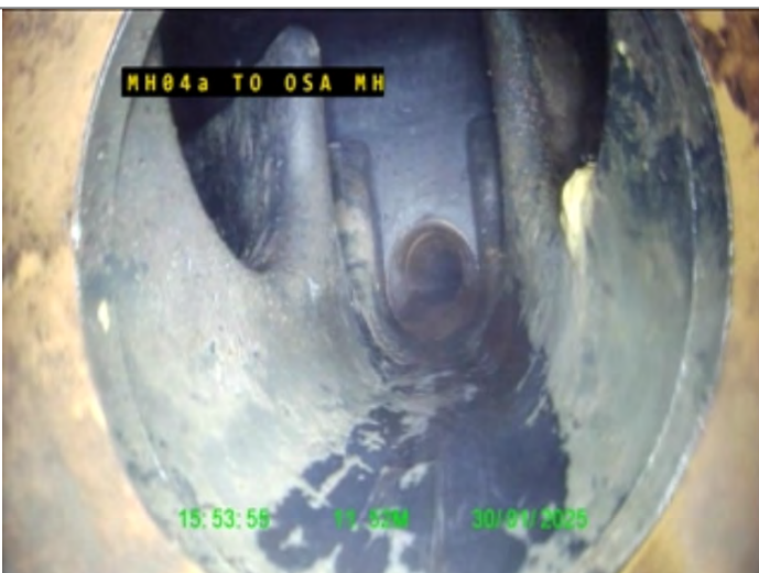
Finish node type, manhole, reference MH OSA
