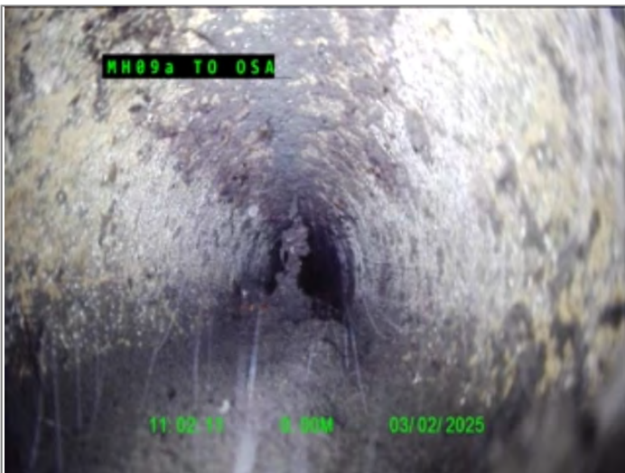
Settled deposits fine 30% cross-sectional area loss
