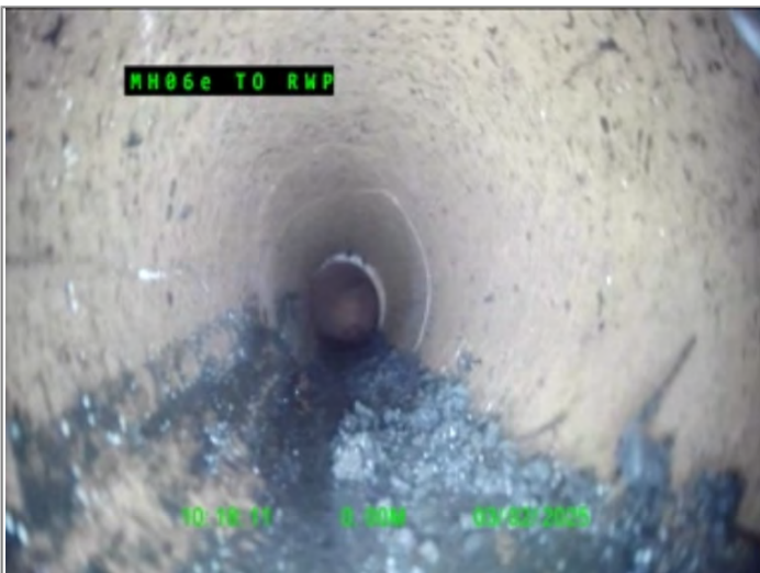
Settled deposits fine 5% cross-sectional area loss, Start
