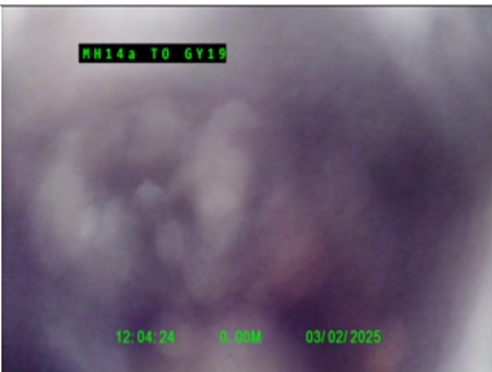
Loss of vision, silt
