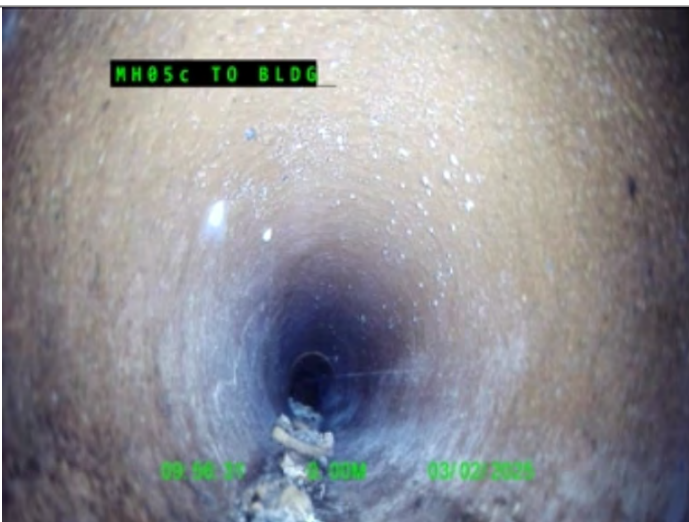
Settled deposits coarse 5% cross-sectional area loss, Start
