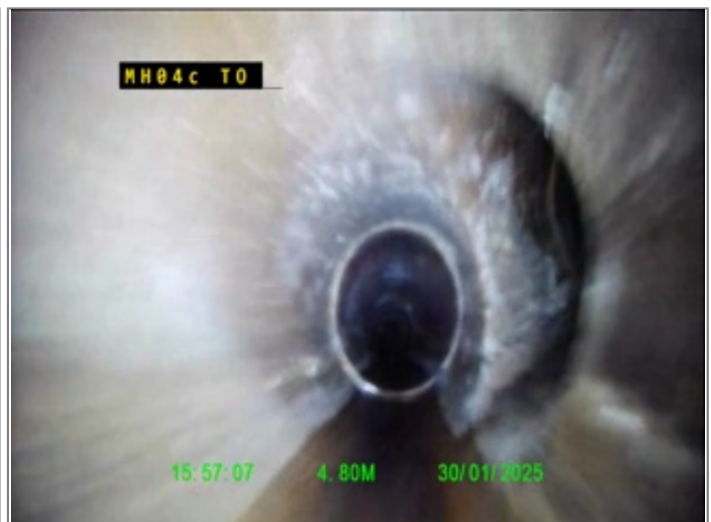
Connection other than junction at 3 o'clock, diameter 100mm
