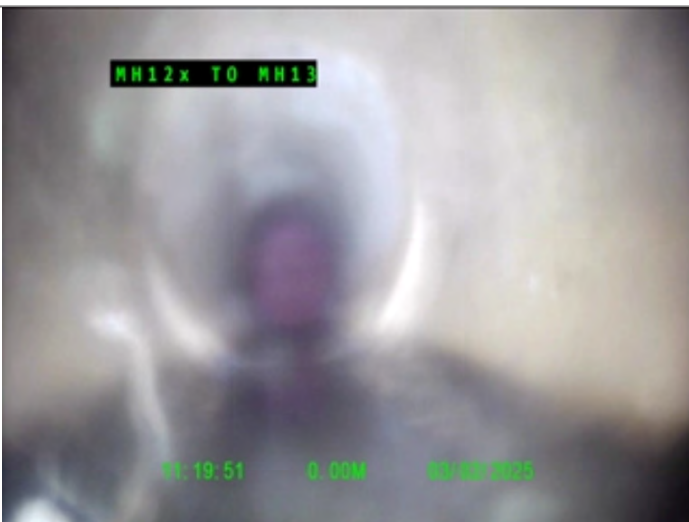
Settled deposits fine 5% cross-sectional area loss
