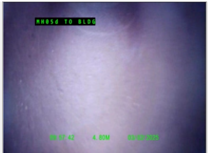
Line of drain/sewer deviates up
