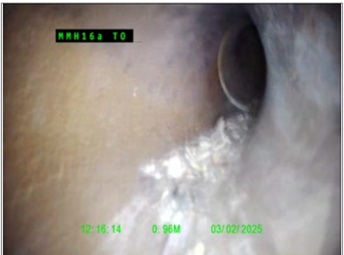
Settled deposits coarse 10% cross-sectional area loss
