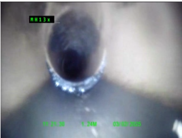
Joint displaced 5mm
