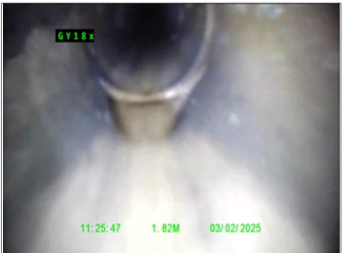
Line of drain/sewer deviates up
