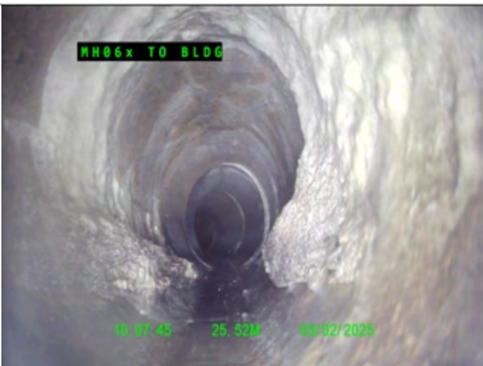
Attached deposits, encrustation at 4 o'clock 5% cross-sectional area loss
