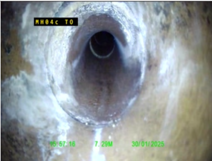
Line of drain/sewer deviates up
