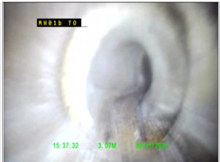
Joint displaced 10mm
