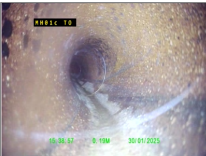
Line of drain/sewer deviates left
