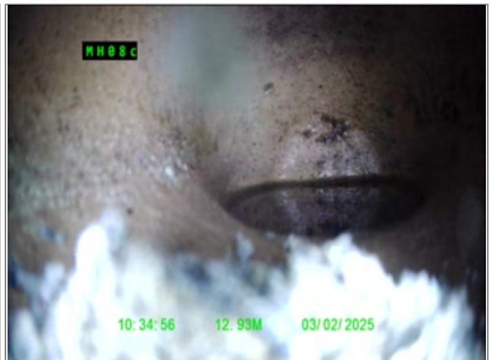
Line of drain/sewer deviates down
