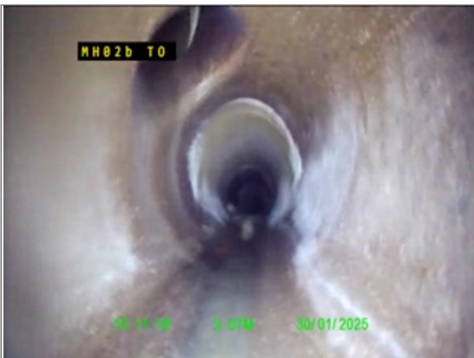
Connection other than junction at 11 o'clock, diameter 100mm
