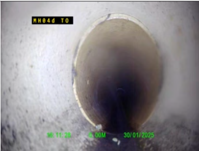
Start node type, Manhole, reference MH04d
