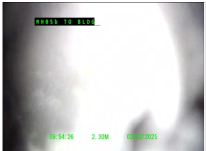
Line of drain/sewer deviates left
