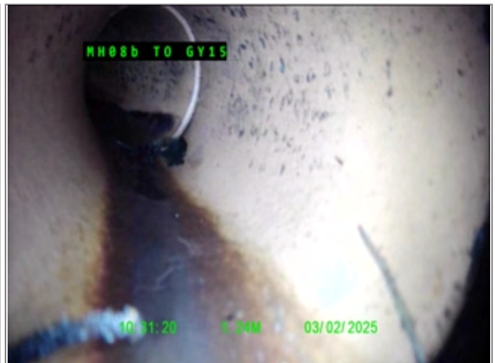
Line of drain/sewer deviates left
