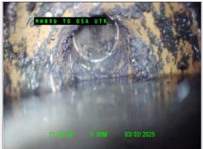
Line of drain/sewer deviates up
