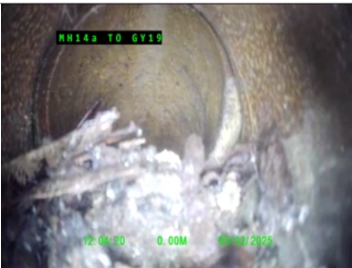
Settled deposits coarse 20% cross-sectional area loss
