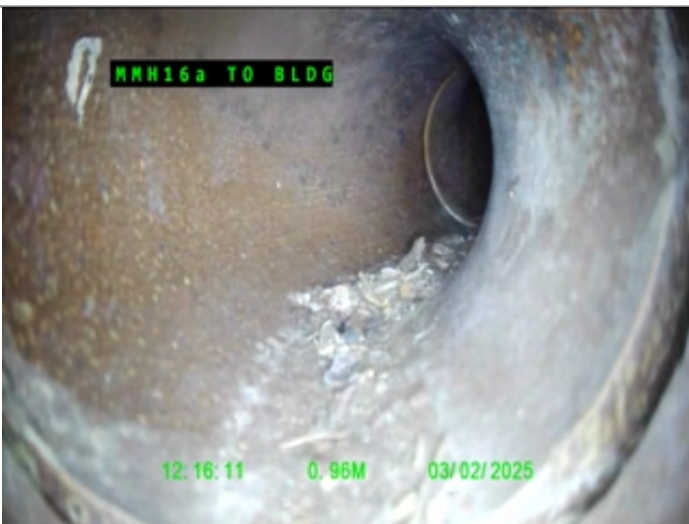
Line of drain/sewer deviates right
