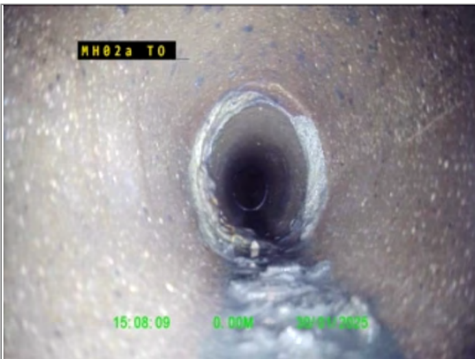
Settled deposits fine 5% cross-sectional area loss
