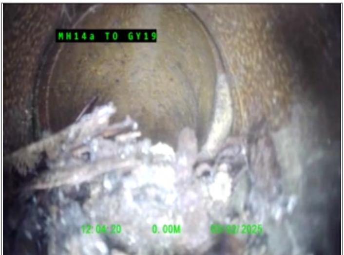
Line of drain/sewer deviates down
