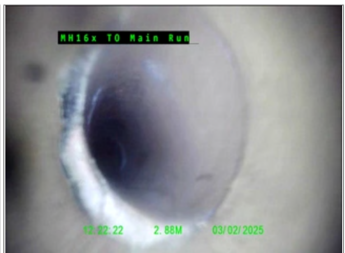
Joint displaced 10mm
