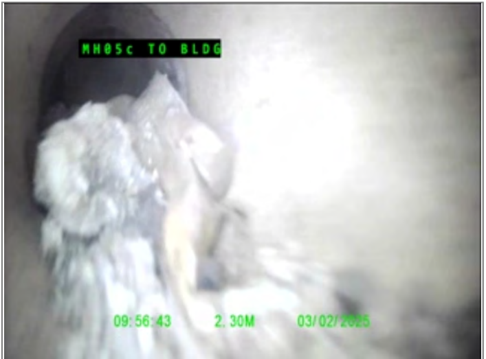
Settled deposits hard or compacted 50% cross-sectional area loss
