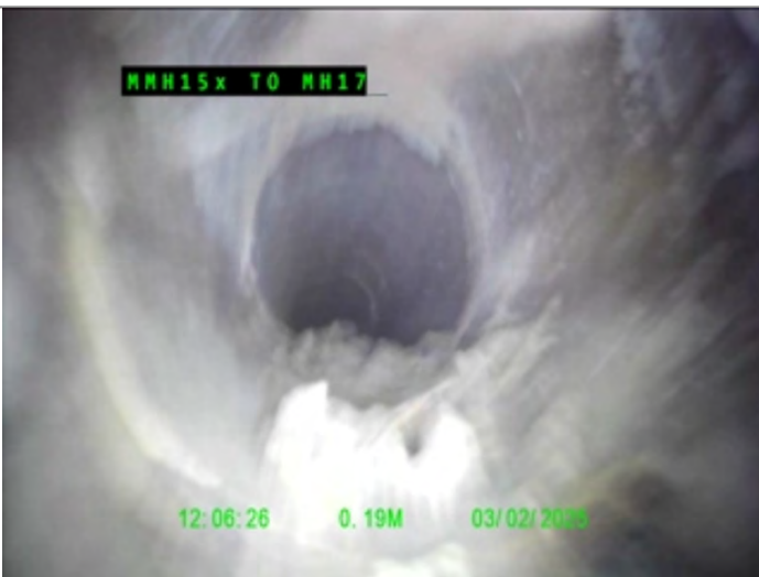
Settled deposits fine 10% cross-sectional area loss
