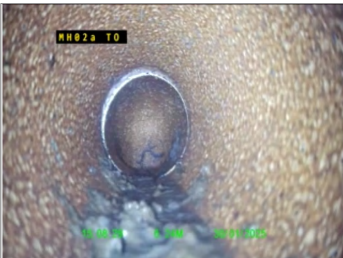
Settled deposits fine 5% cross-sectional area loss
