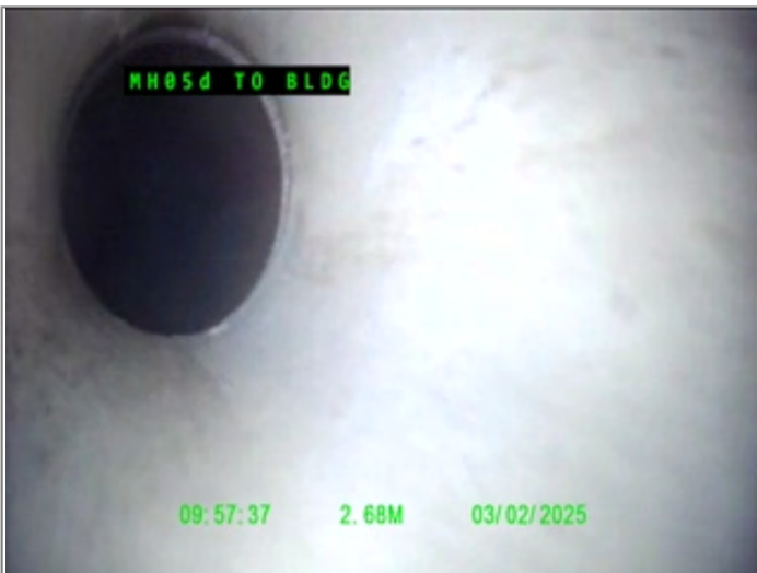
Line of drain/sewer deviates left
