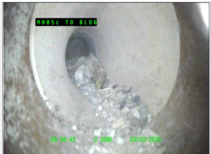
Settled deposits coarse 5% cross-sectional area loss, Finished
