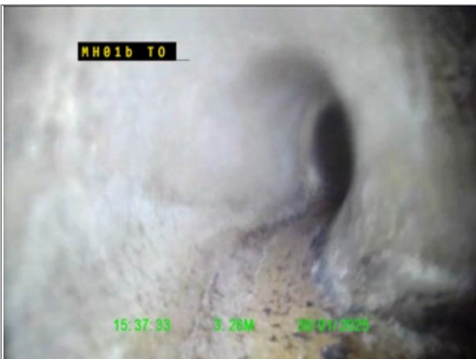
Line of drain/sewer deviates right
