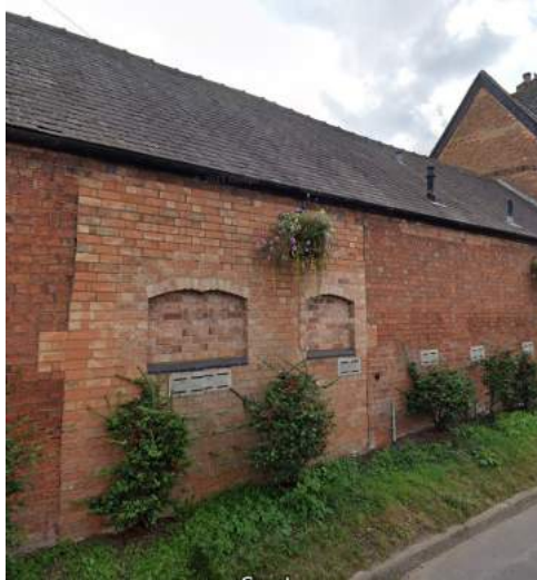
Recessed Brick Detail - Old Manor House
