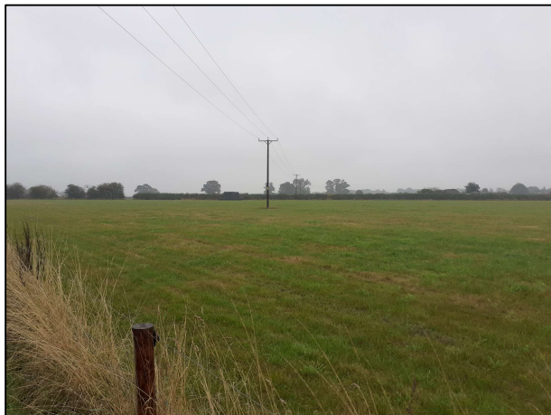
Photo 11: View looking east at the overhead electricity cables in the south.
