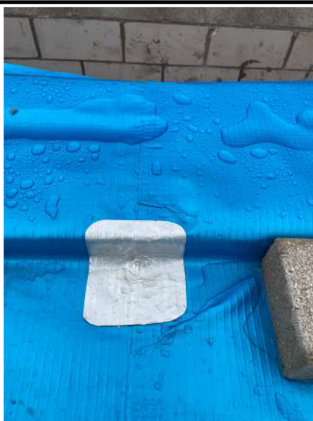
A patch of Visqueen GR SAM which has been used to seal a fault identified.
