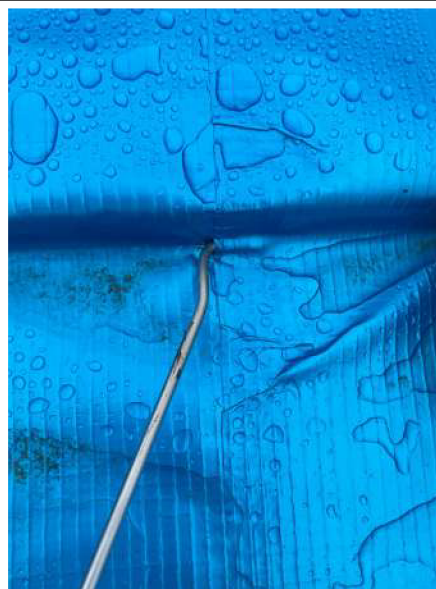
A probe demonstrating a fault identified.
