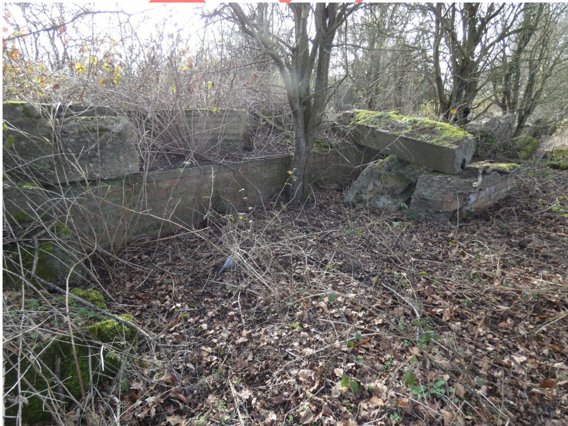
Figure 26: Collapsed walls and rubble found on the western side of the platform.
