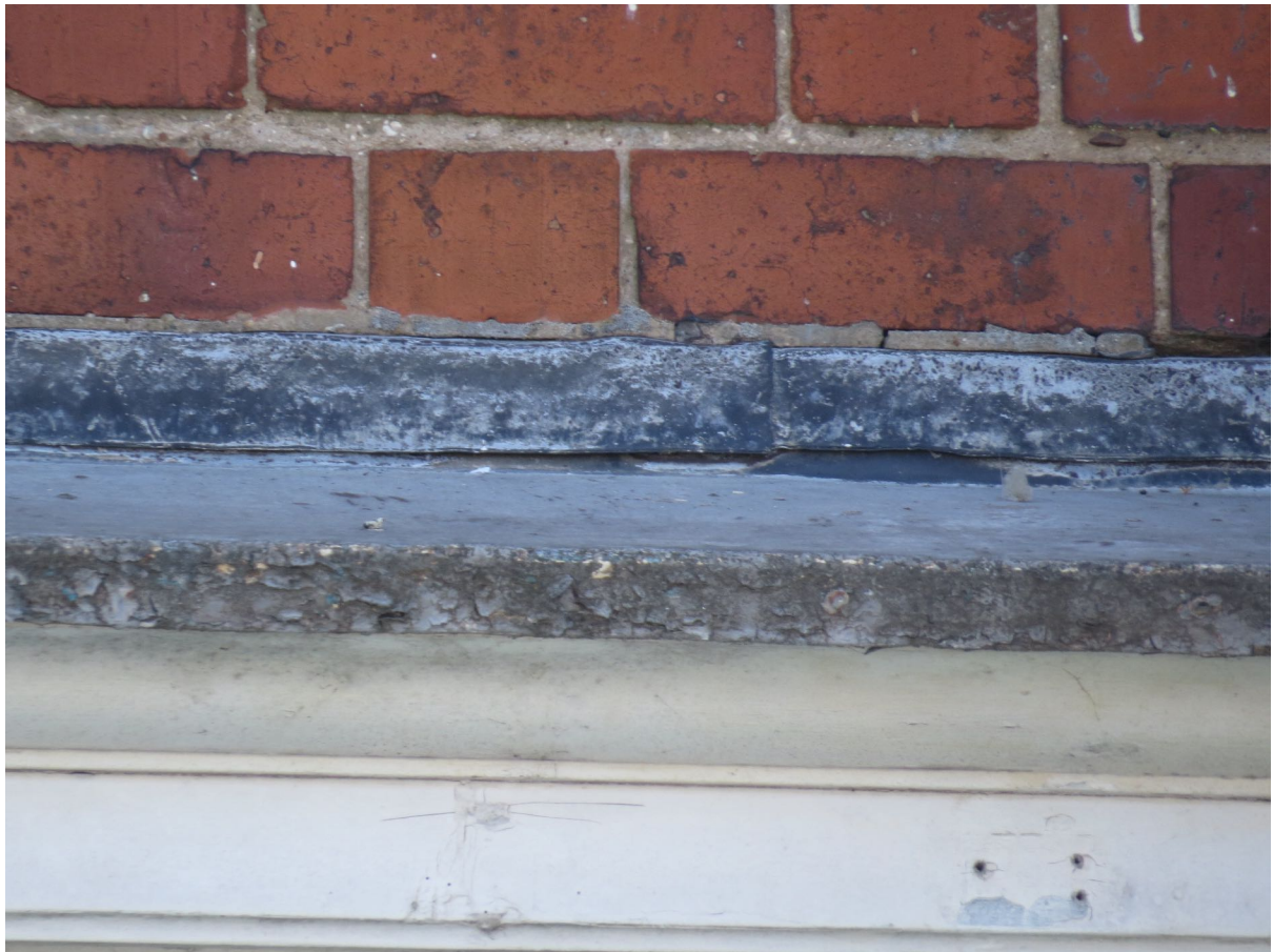
5 – Lead flashing above signage is fitted tightly with no suitable gaps.
