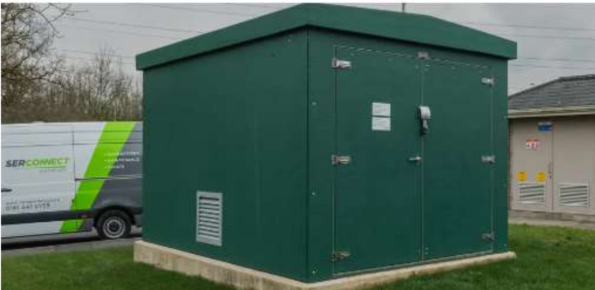
Photograph of typical substation and housing.
