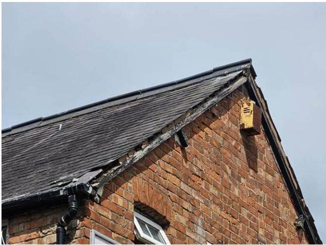
Gaps in south eaves of western building
